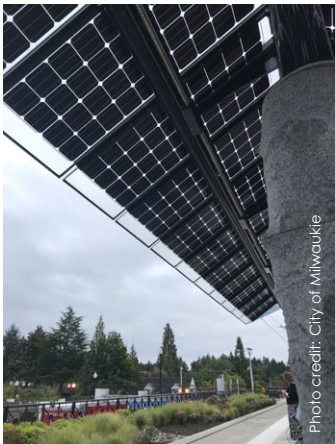
Solar panels at MAX Station
