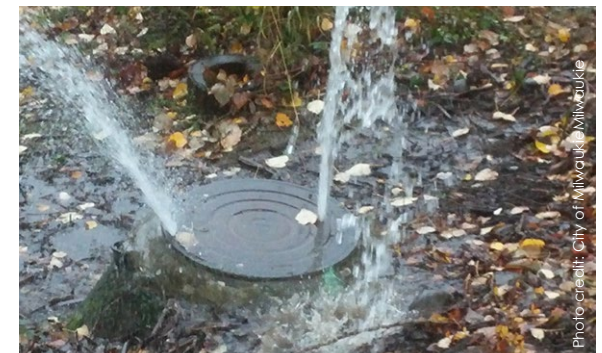
Storm drain surcharge in 2015
