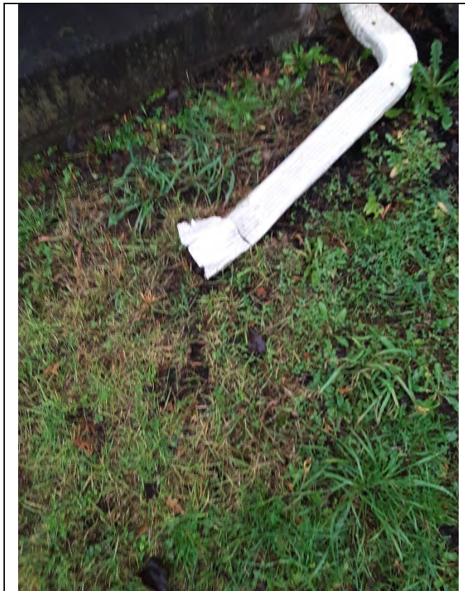
BUILDING EXTERIOR – DAMAGED DOWNSPOUT
