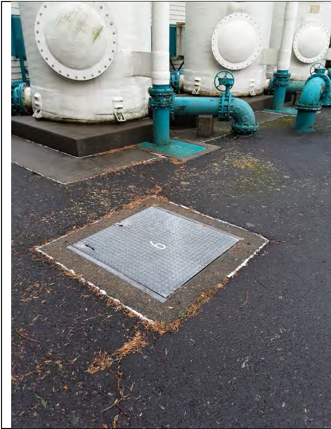
TP235 AIR STRIPPING TOWER SITE
