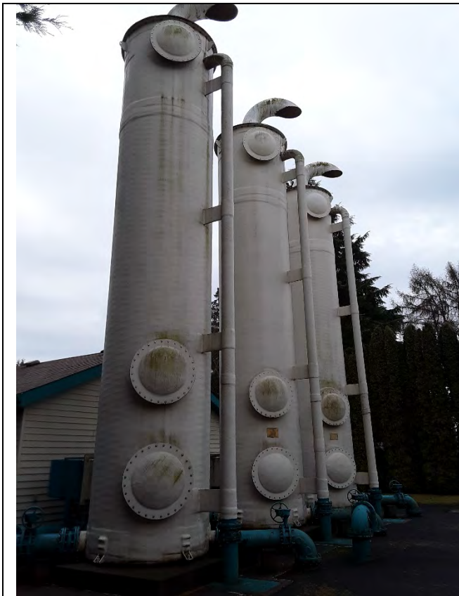
TP235 AIR STRIPPING TOWERS
