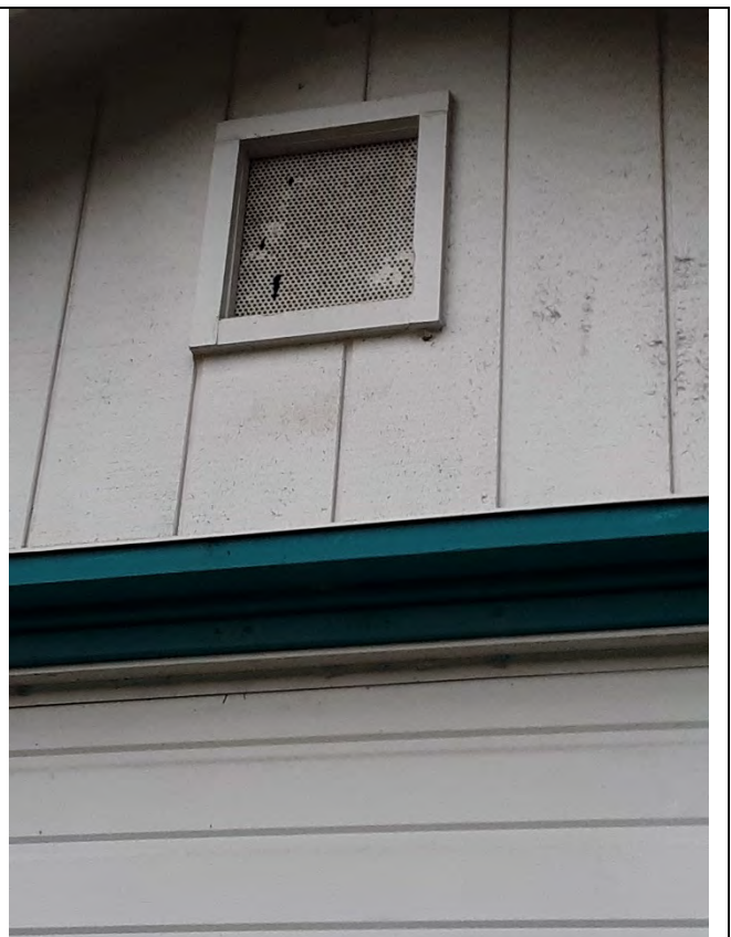
BUILDING EXTERIOR – DAMAGED SCREEN
