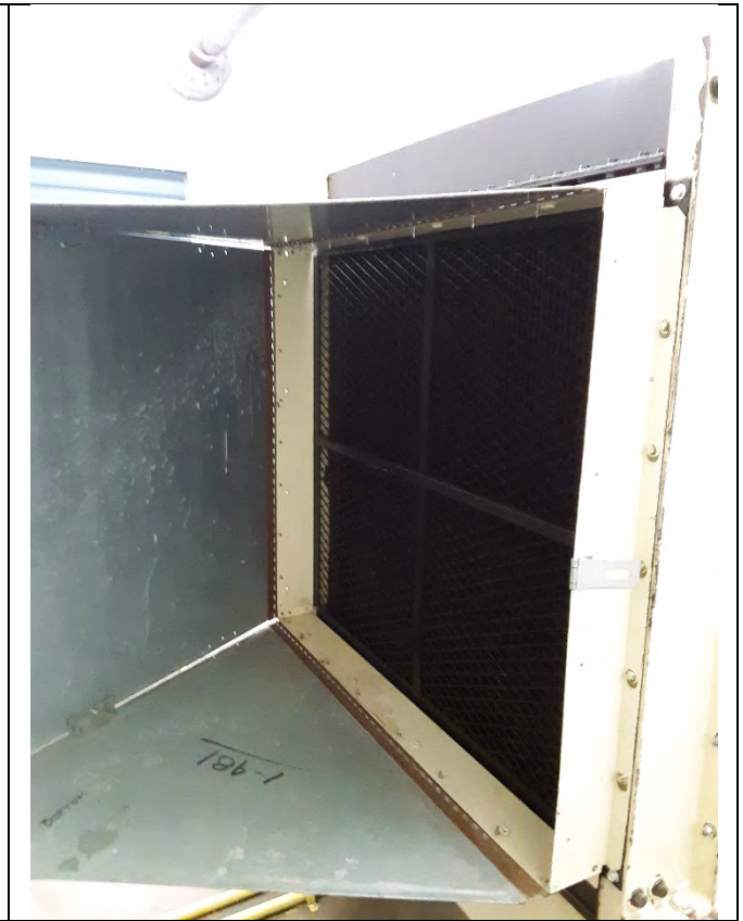
EMERGENCY GENERATOR EXHAUST
