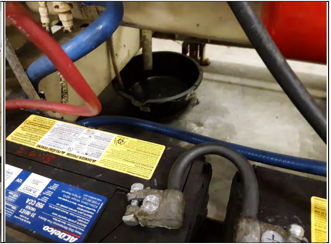
EMERGENCY GENERATOR – LEAK
