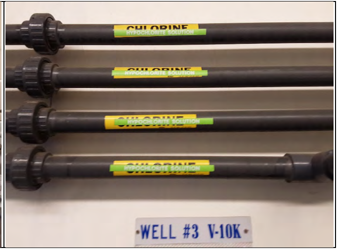
TP235 CHLORINE FEED SYSTEM
