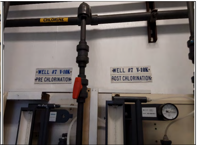
TP37 CHLORINE INJECTION SYSTEM
