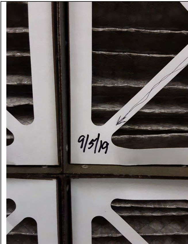
TP47 BLOWER ROOM AIR FILTERS
