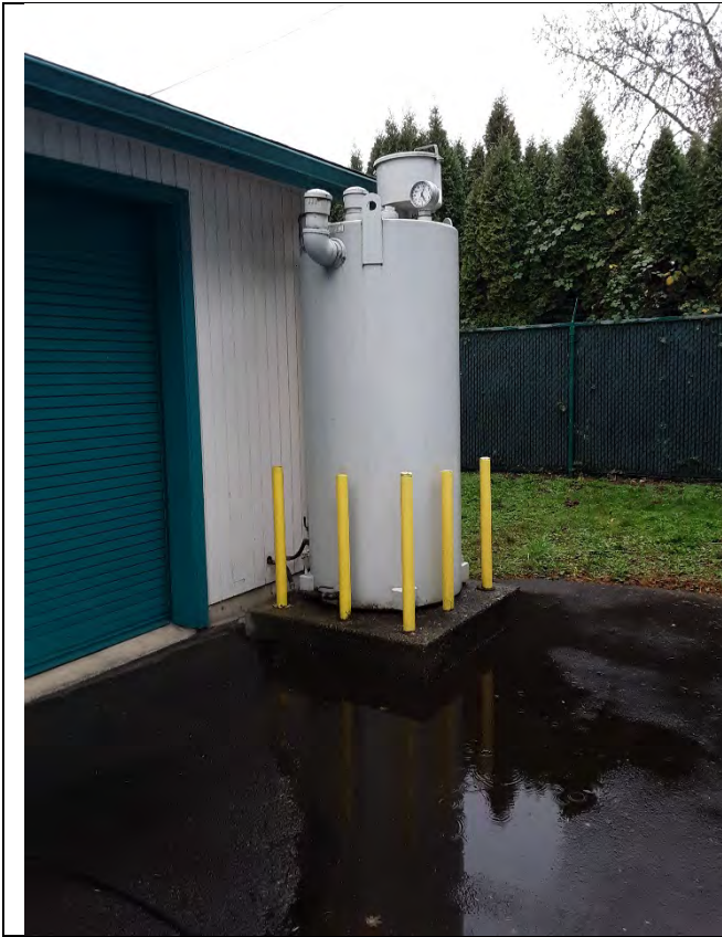
FIRE PUMP DIESEL TANK
