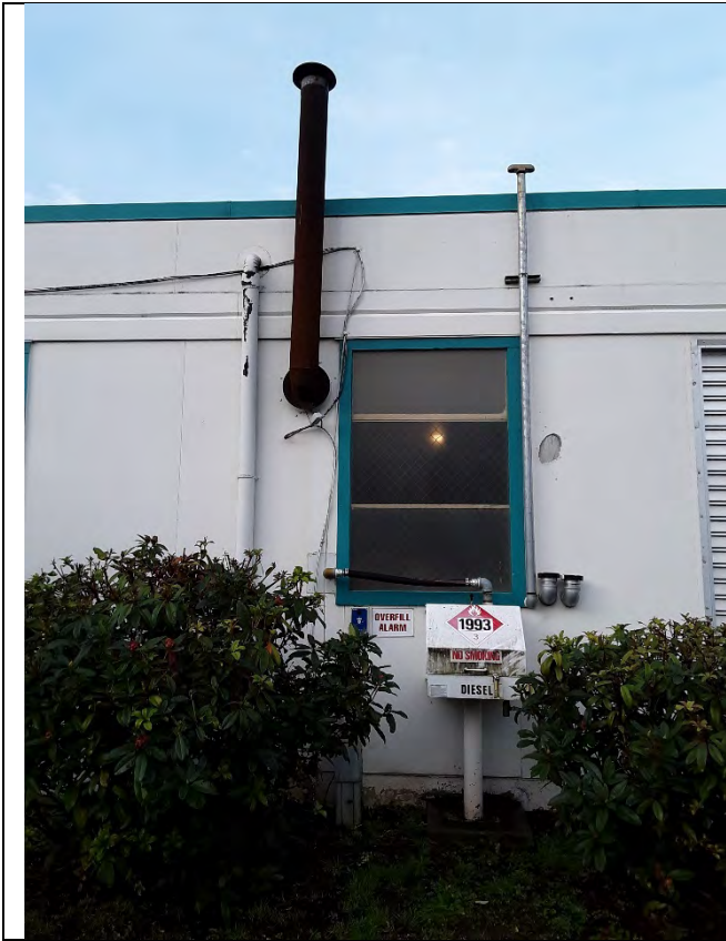
GENERATOR DIESEL FILL TAP
