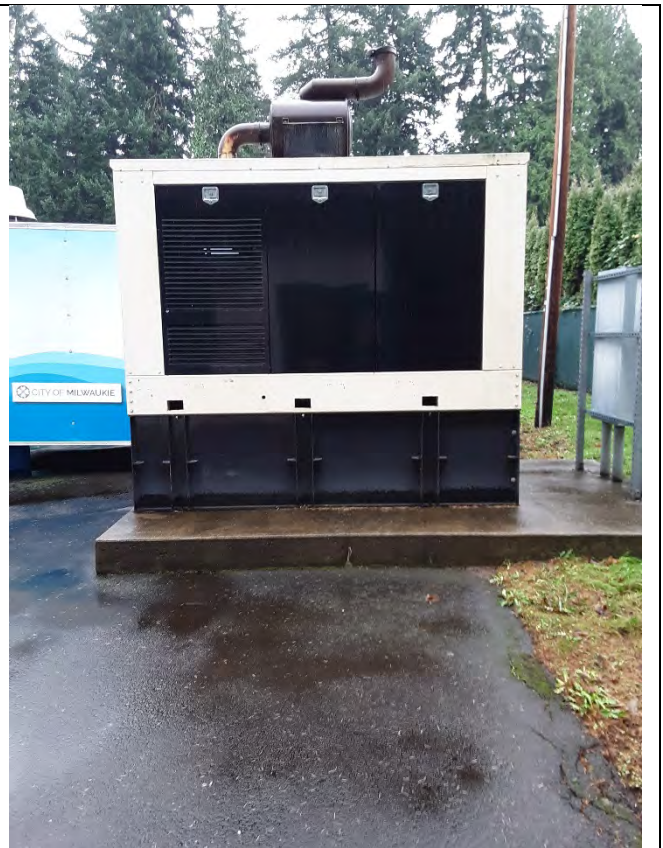
STANDBY EMERGENCY GENERATOR
