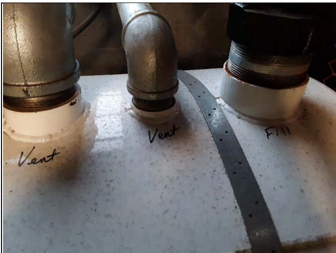
TP235 GENERATOR – DIESEL STORAGE
