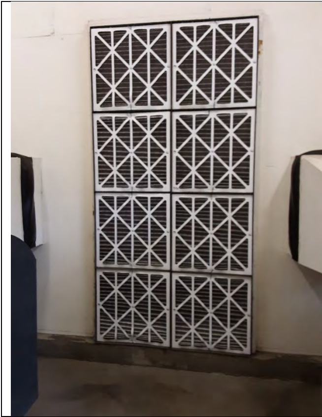
TP47 BLOWER ROOM AIR FILTERS
