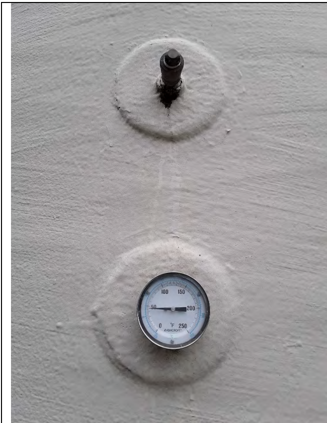
TP235 AIR STRIPPING TOWER GAUGE
