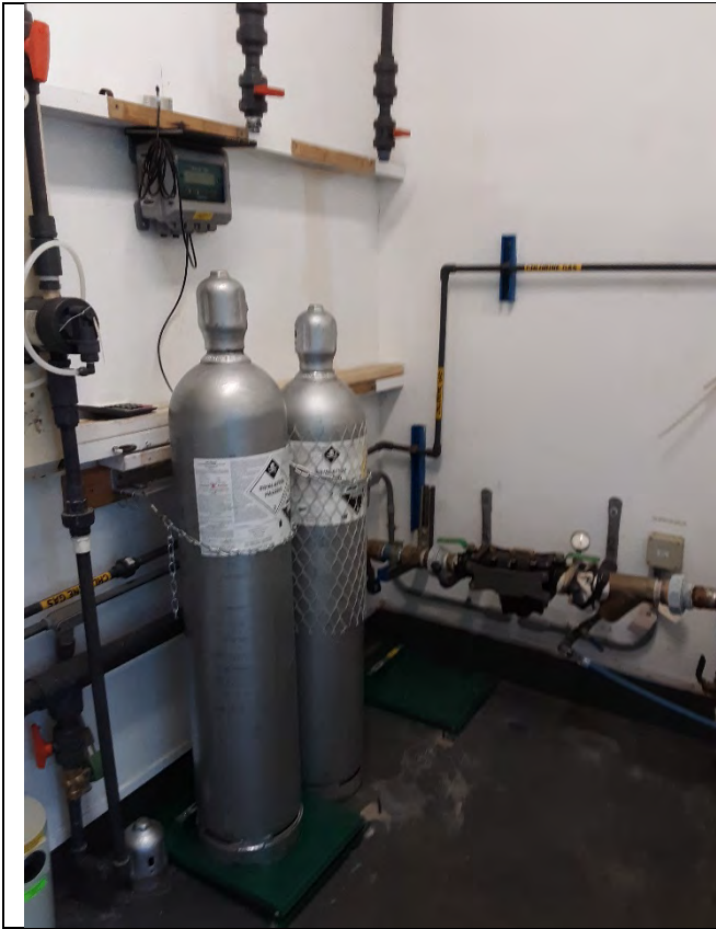
TP47 CHLORINE TANKS
