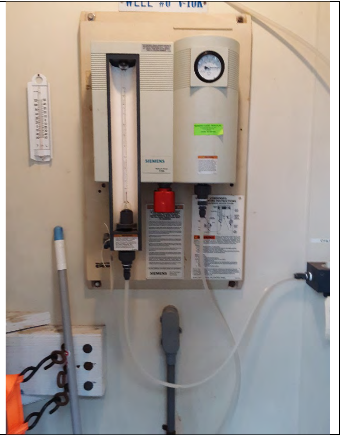
CHLORINE INJECTION SYSTEM
