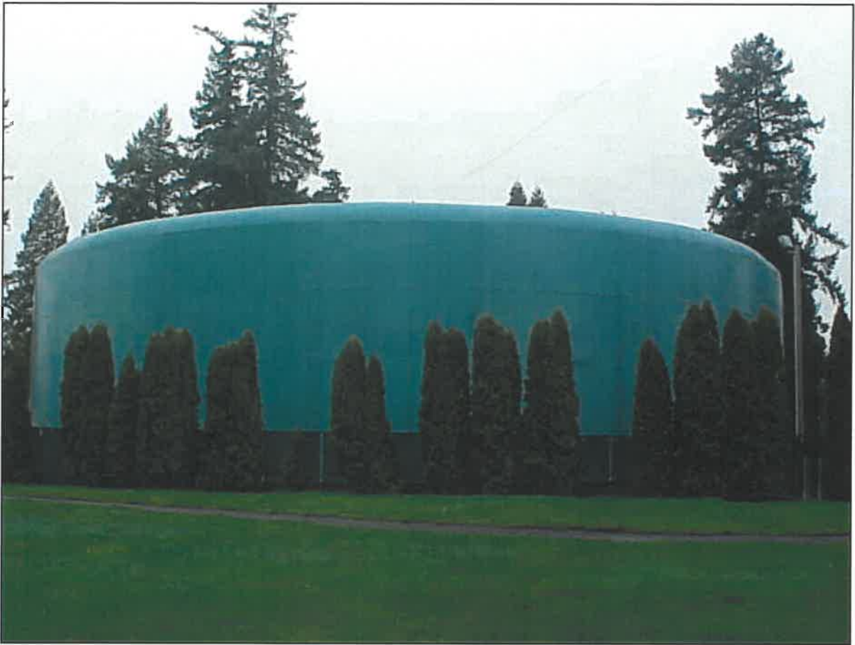
Stanley Avenue Reservoir 3.0 million gallons
