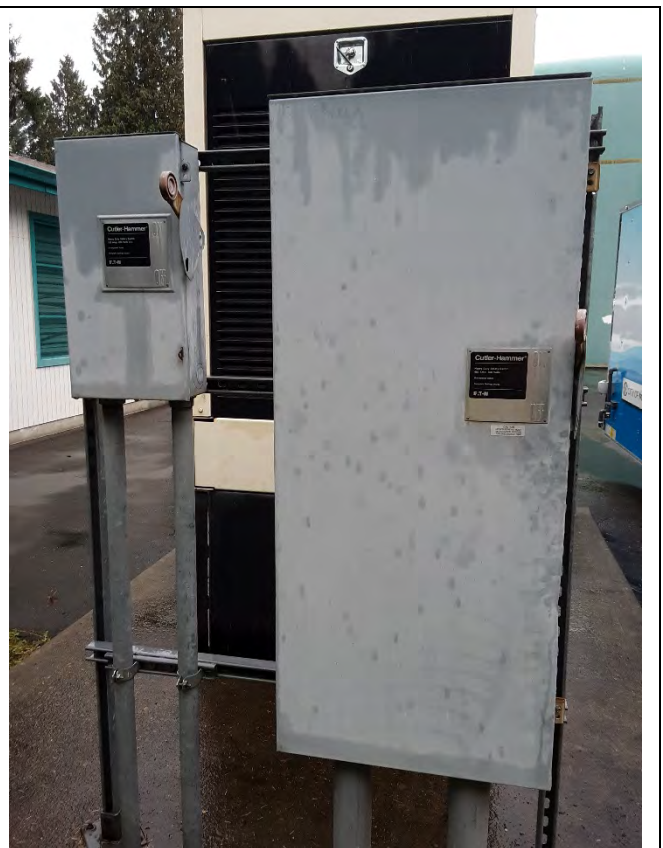
AUTOMATIC TRANSFER SWITCH
