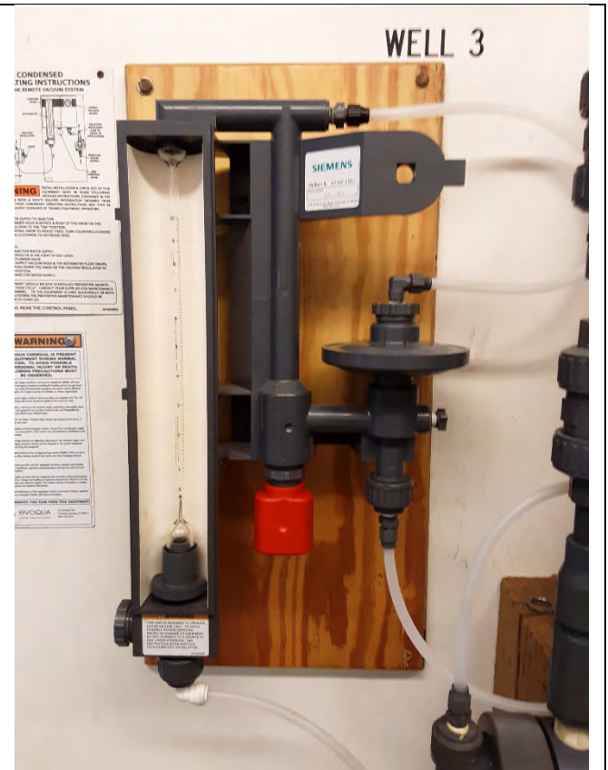
TP235 CHLORINE FEED SYSTEM
