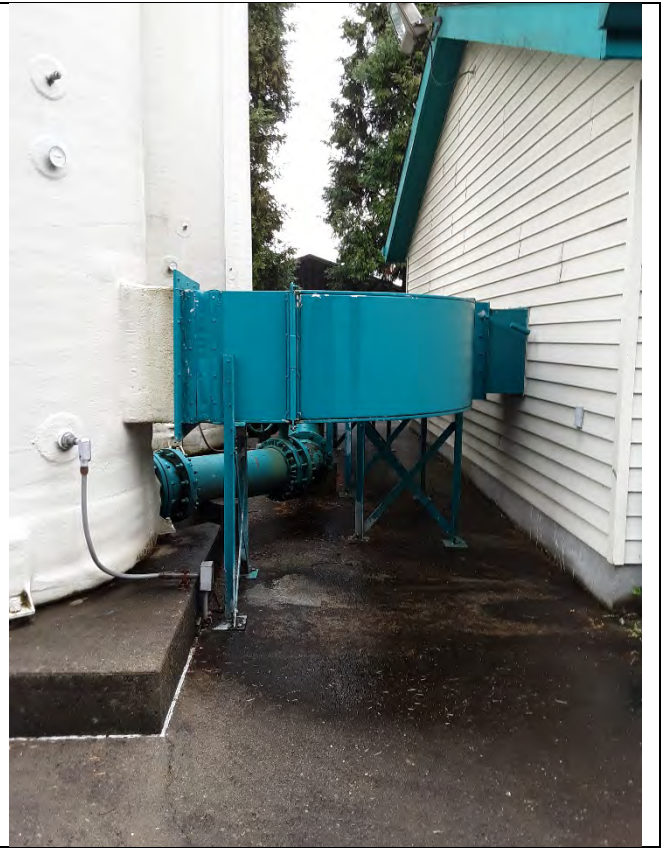
TP235 AIR STRIPPING TOWERS
