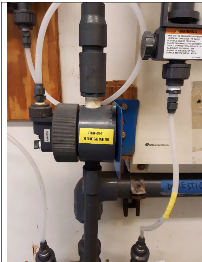
TP235 CHLORINE FEED SYSTEM
