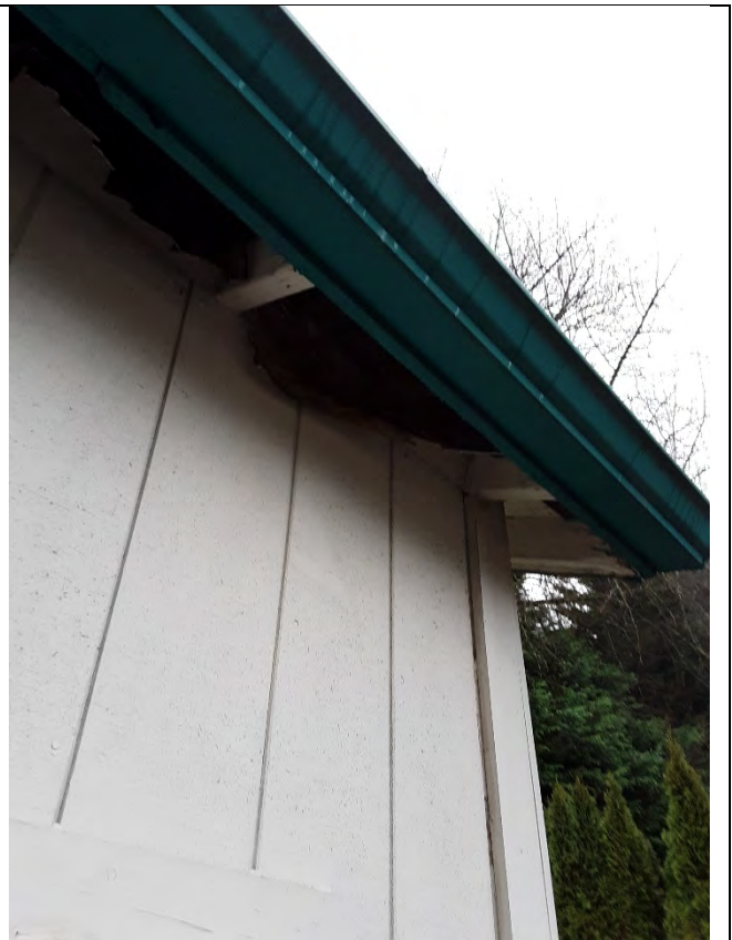
BUILDING EXTERIOR – DEFERRED MAINTENANCE
