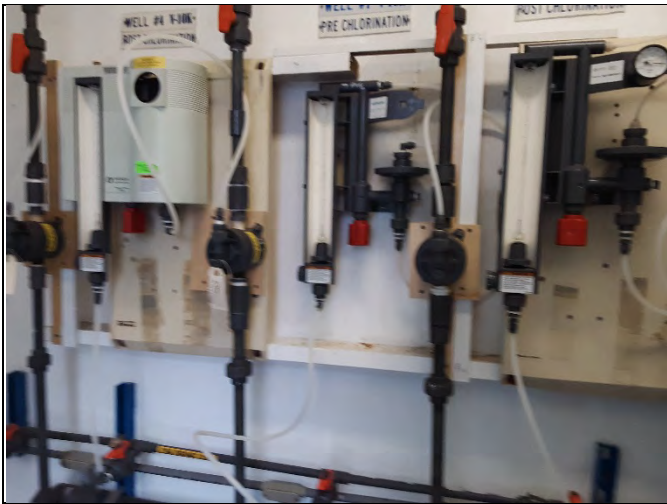
TP37 CHLORINE INJECTION SYSTEM
