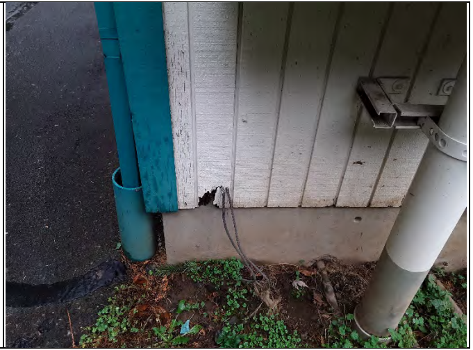
BUILDING EXTERIOR – DEFERRED MAINTENANCE SIDING
