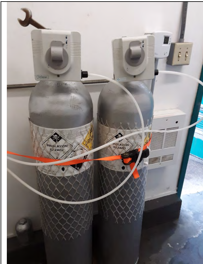
TP47 CHLORINE STORAGE
