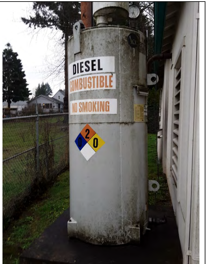
GENERATOR DIESEL STORAGE
