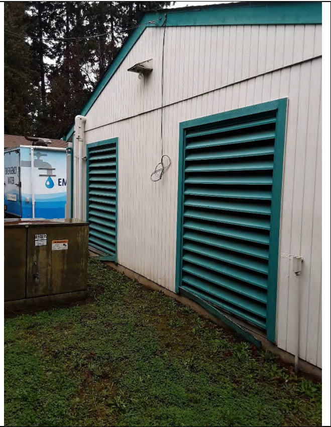
BUILDING EXTERIOR – DEFERRED MAINTENANCE LOUVERS
