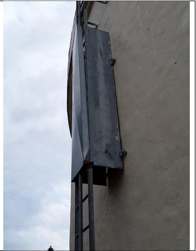
CONCRETE RESERVOIR LADDER COVER DAMAGE
