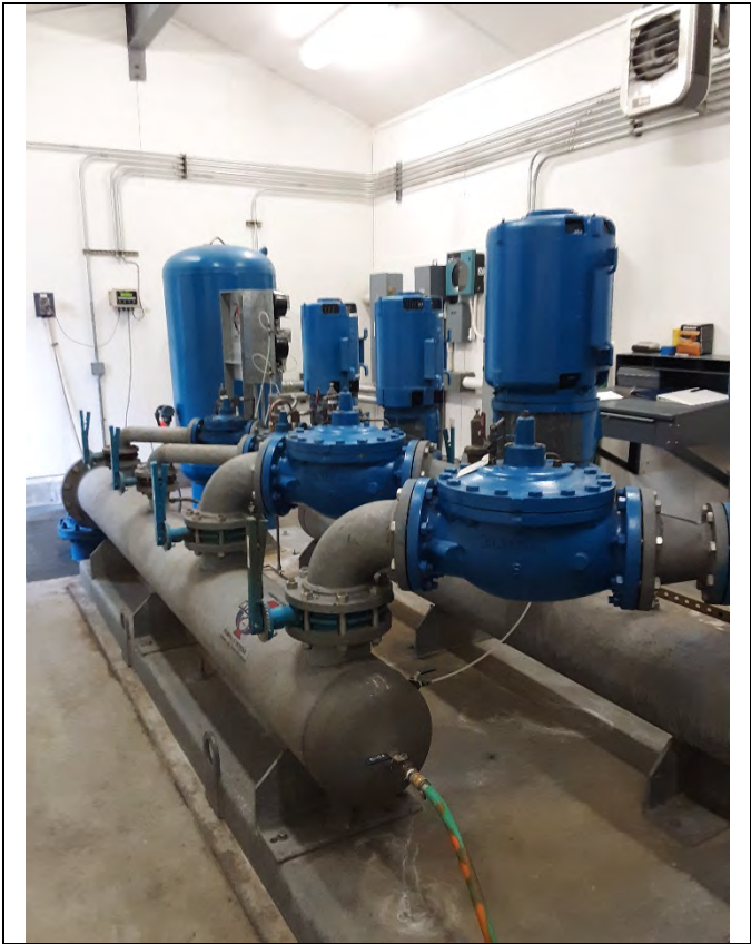
PRESSURE ZONE 3 BOOSTER PUMPS
