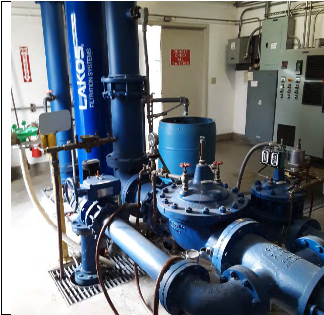
SAND FILTER AND BACKWASH
