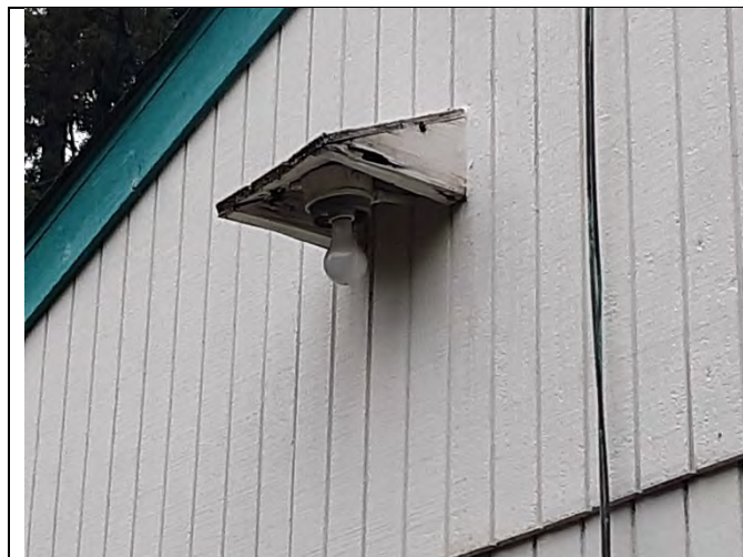
BUILDING EXTERIOR – DEFERRED MAINTENANCE LIGHTING
