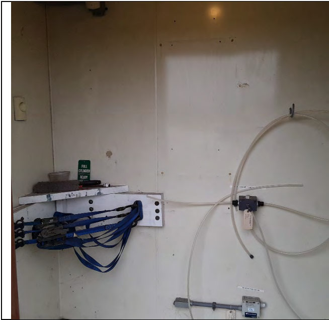
CHEMICAL FEED ROOM
