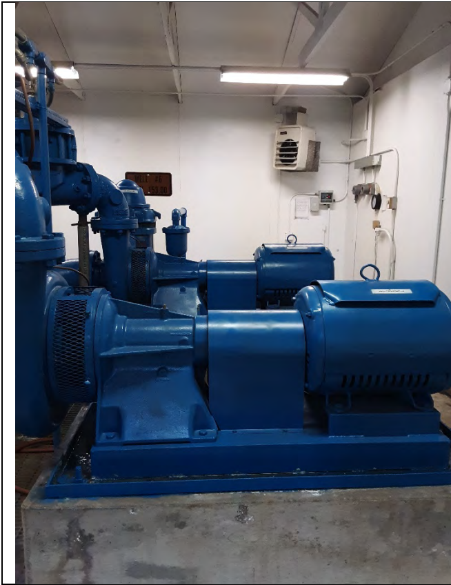
WELL 6 TRANSFER PUMPS
