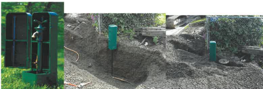
Typical installation of Eclipse #88 sample station
