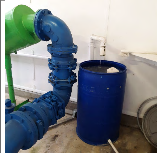
SAND FILTER AND BACKWASH
