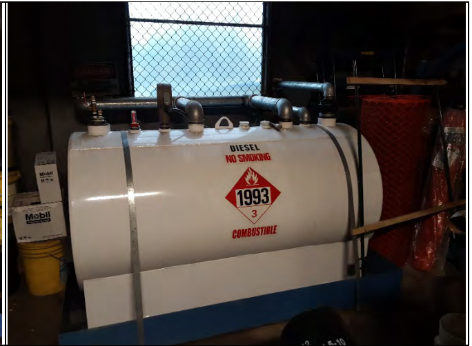
TP235 GENERATOR – DIESEL STORAGE
