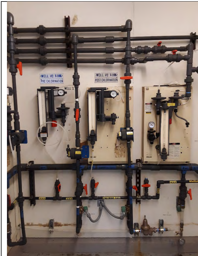
TP235 CHLORINE FEED SYSTEM
