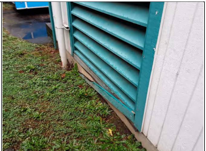
BUILDING EXTERIOR – DEFERRED MAINTENANCE LOUVERS
