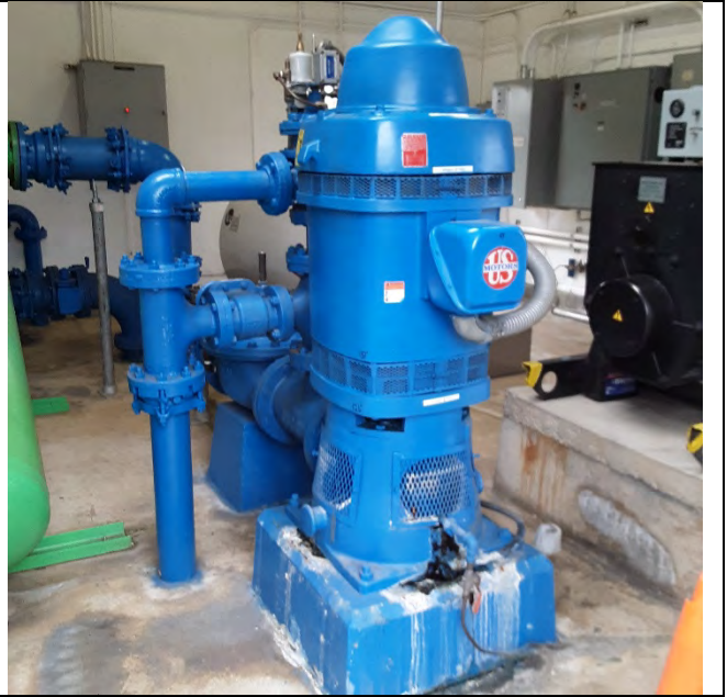
WELL NO. 6 PUMP
