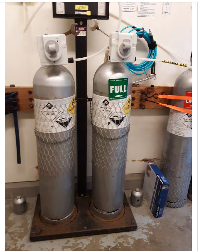
TP235 CHLORINE TANKS AND SCALE
