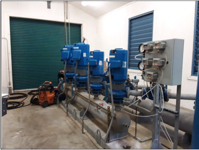
PRESSURE ZONE 3 BOOSTER PUMPS
