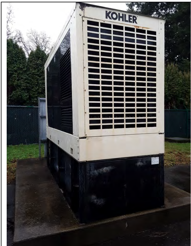
STANDBY EMERGENCY GENERATOR
