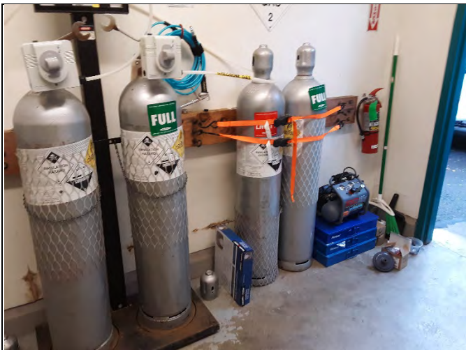
TP235 CHLORINE FEED IN USE AND SUPPLY
