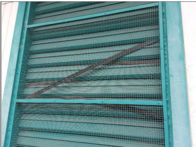
BUILDING EXTERIOR – DEFERRED MAINTENANCE LOUVERS
