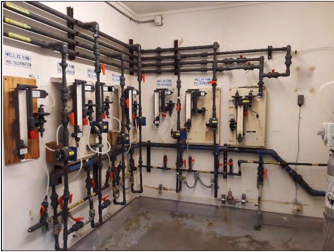
TP235 CHLORINE FEED SYSTEM
