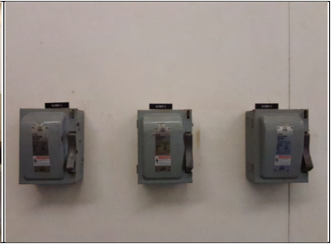
TP235 BLOWER SWITCHES
