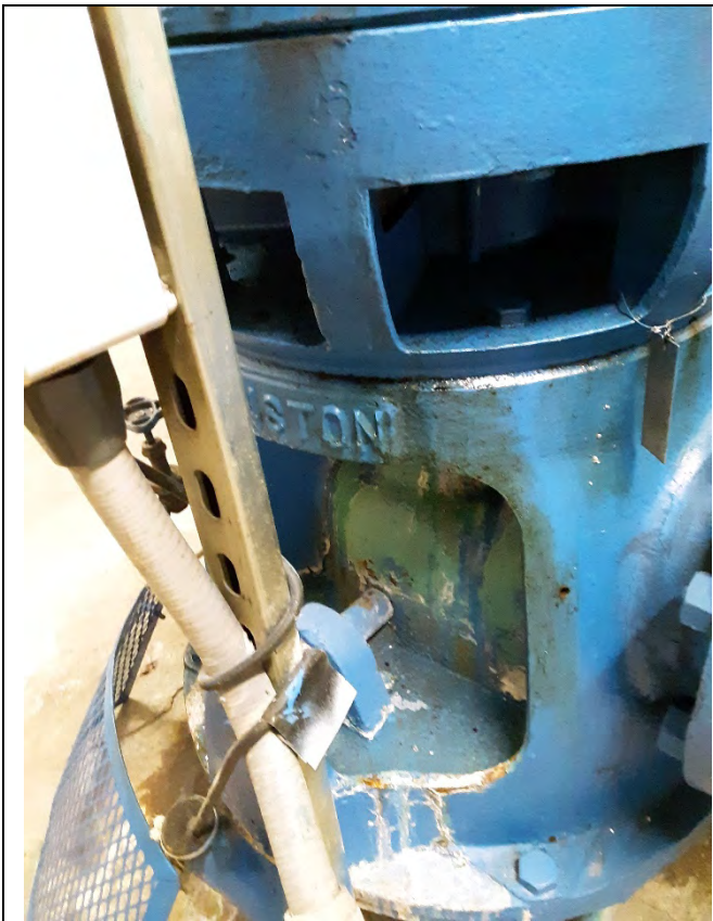
WELL 5 PUMP - LEAK
