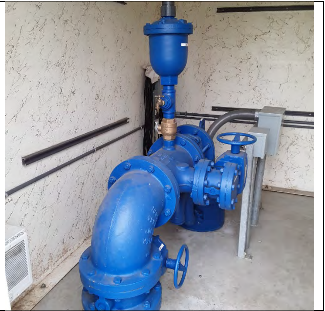
WELL NO. 8 PUMP
