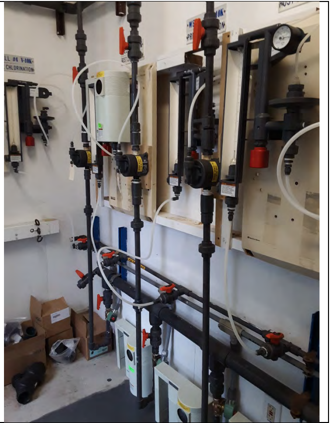
TP37 CHLORINE INJECTION SYSTEM
