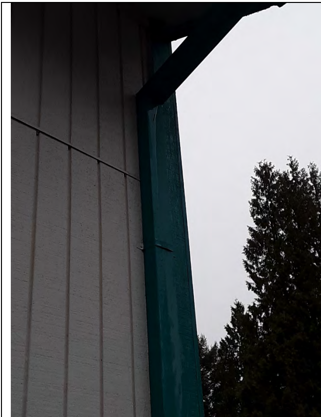
BUILDING EXTERIOR – DEFERRED MAINTENANCE GUTTER
