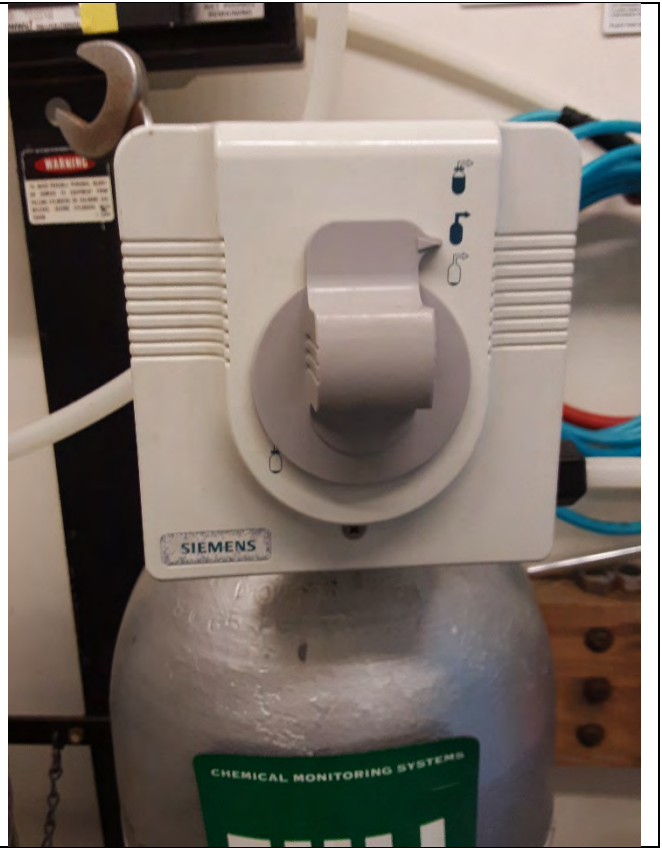
CHLORINE FLOW VALVE
