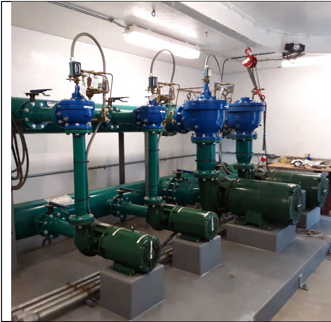
BOOSTER PUMPS AND HIGH DEMAND PUMPS
