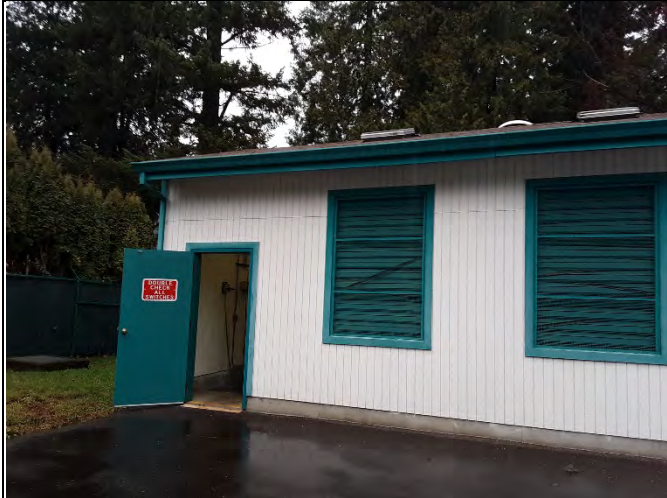
BUILDING EXTERIOR – DEFERRED MAINTENANCE LOUVERS
