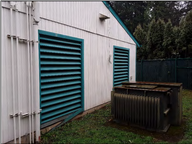
BUILDING EXTERIOR – DEFERRED MAINTENANCE LOUVERS
