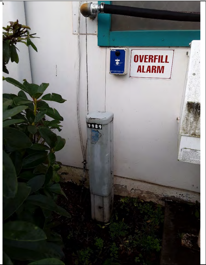
GENERATOR DIESEL FILL TAP
