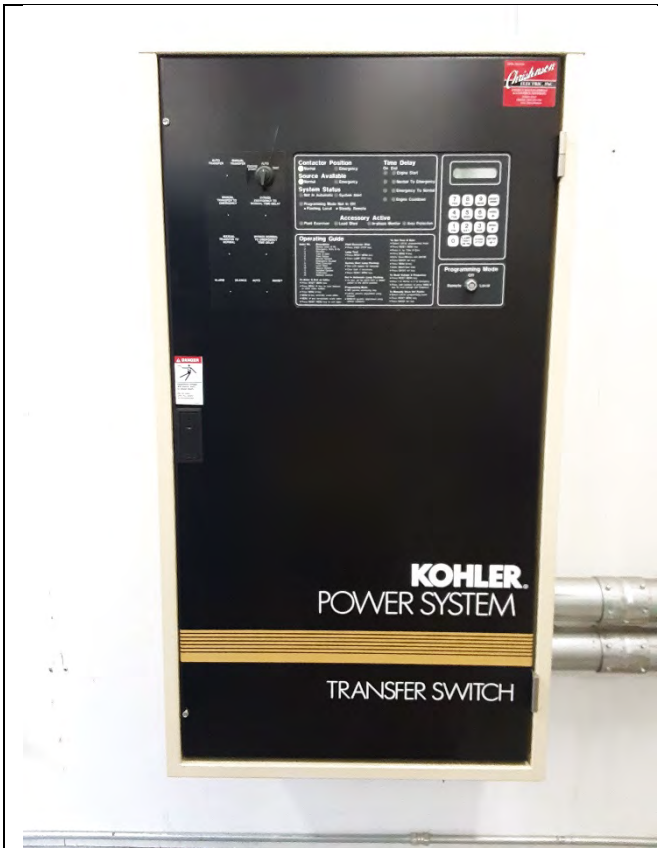
AUTOMATIC TRANSFER SWITCH
