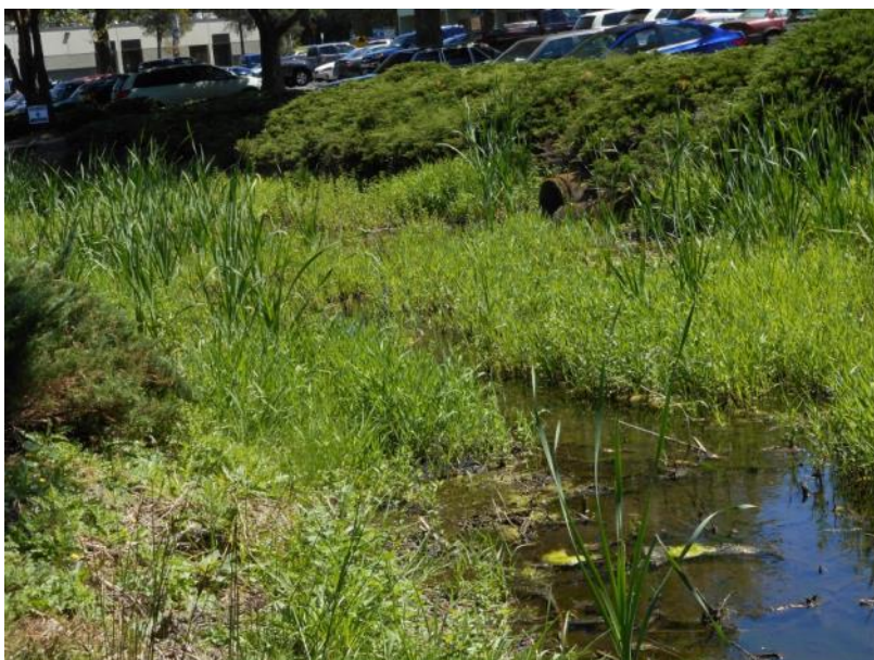
Site location: 007 Photo number: 044 Description: Roof drain and parking lot runoff directly discharges to channel.
