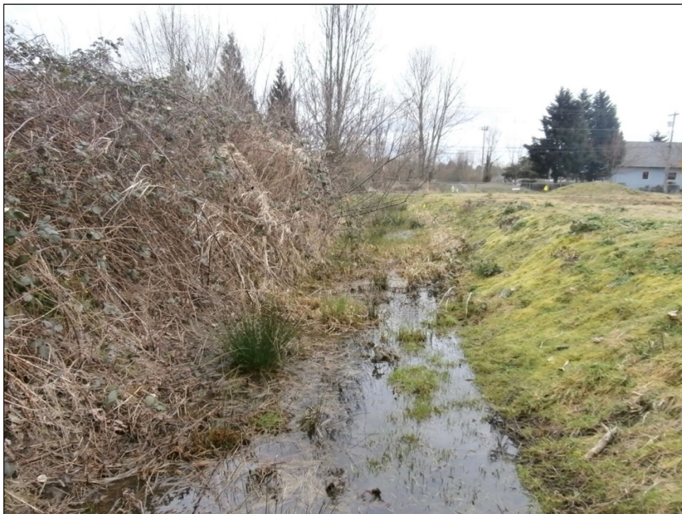
Photo B. View east of the detention pond constructed in 2002, and the berm in photo left along the south side of the stream.
