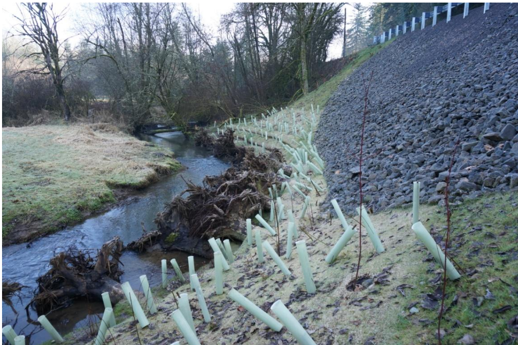
Photo 5: Rock slope stabilization with logs and planting at toe in Clark County, WA. The blue tubes are browse protection for the installed plants.
