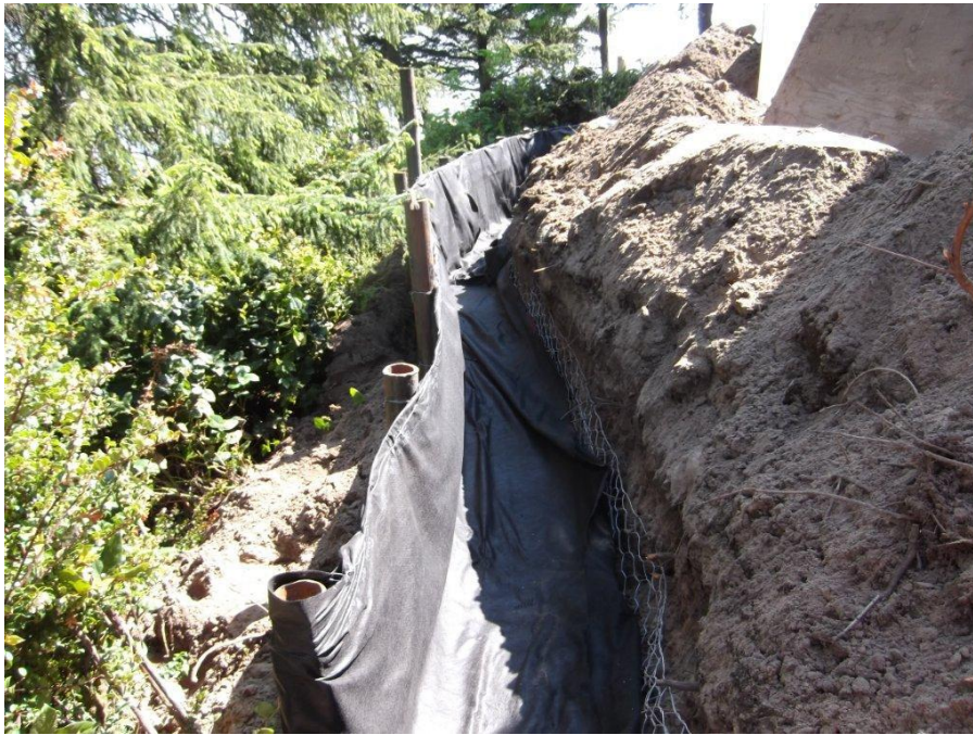
Photo 1: Micropile wall during construction. The wire mesh and fabric reinforce the concrete wall between the piles.
