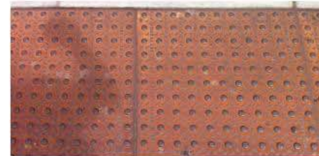
Metal Detectable Warning Panel @ Crosswalks
