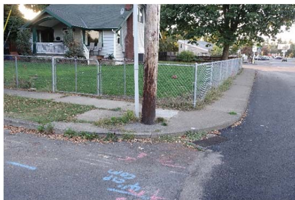
Narrow sidewalk without curb ramps at Campbell Street and Myrtle Street
