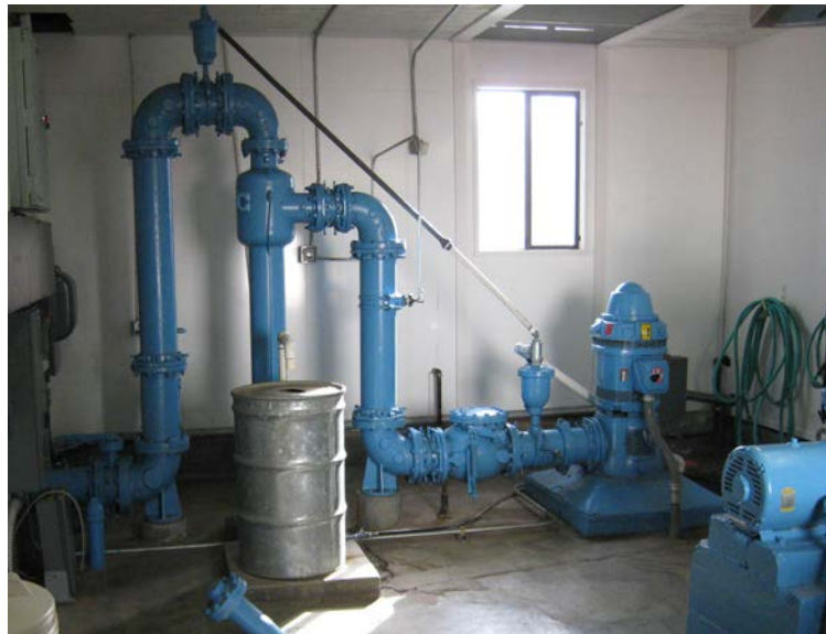
Figure 3-3. Well No. 2, Typical Well Discharge Configuration
