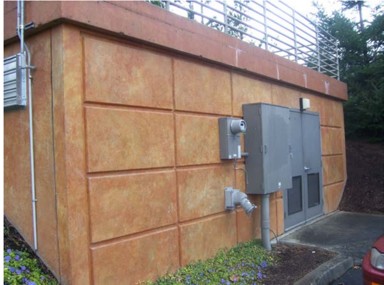
Figure 3-9. Lava Drive Pump Station
