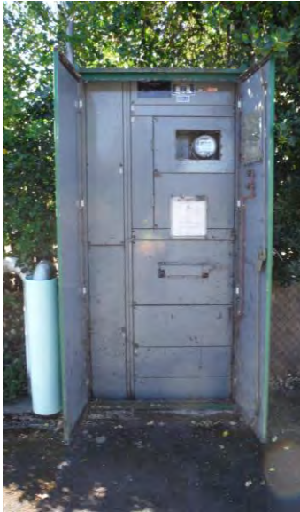
(a) Overall View of Electrical Cabinet
