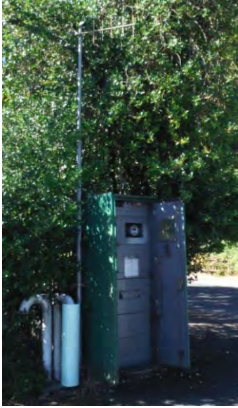
(a) SCADA Antenna
