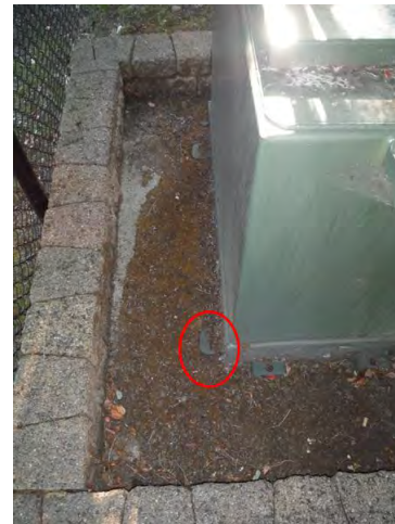
(b) No Anchors between Transformer and Concrete Pad Visible from Exterior of Transformer
