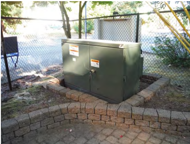
(a) Overall View of Electrical Transformer
