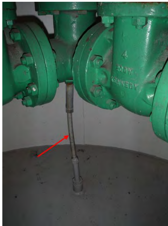
Figure 3.10 – Pipes/Valves Potentially Lacking Adequate Gravity Support
