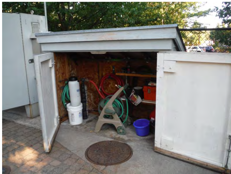
Figure 3.21 – Washdown Water and Storage Enclosure
