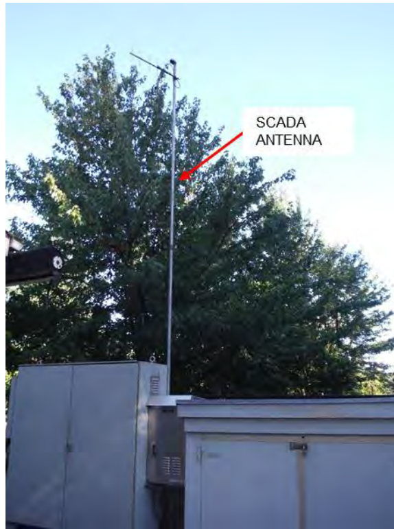
Figure 3.33 – Long Slender SCADA Antenna Mast
