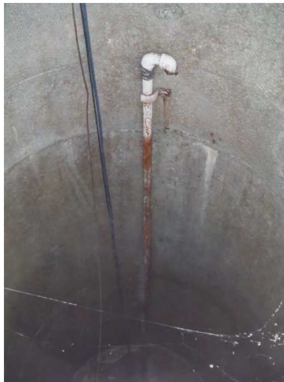
Figure 3.8 – Vertical Pipe in Wet Well not Seismically Braced
