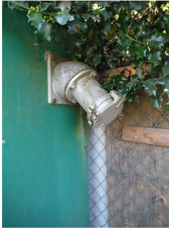
Figure 3.3 – Emergency Generator Hookup on Electrical Cabinet
