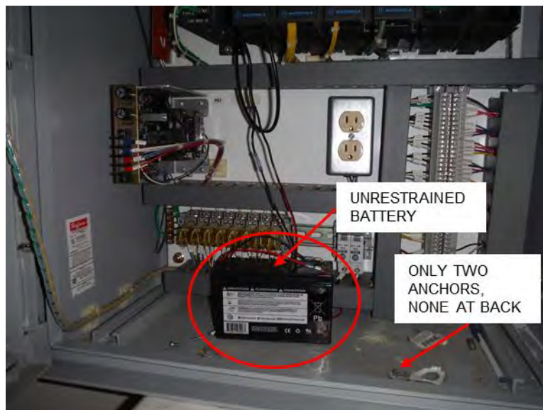
Figure 3.14 – Missing Anchors for SCADA Cabinet and Backup Battery
