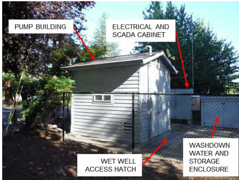
Figure 3.18 – Brookside Lift Station (S5) Components
