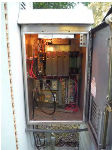
(a) SCADA Cabinet
