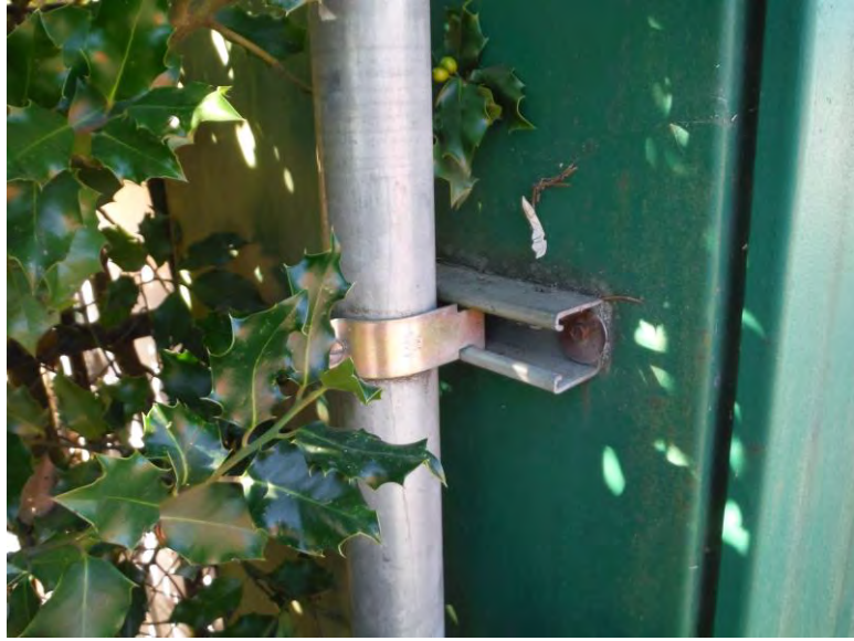
(b) Antenna Mast Supported with Friction Clips
