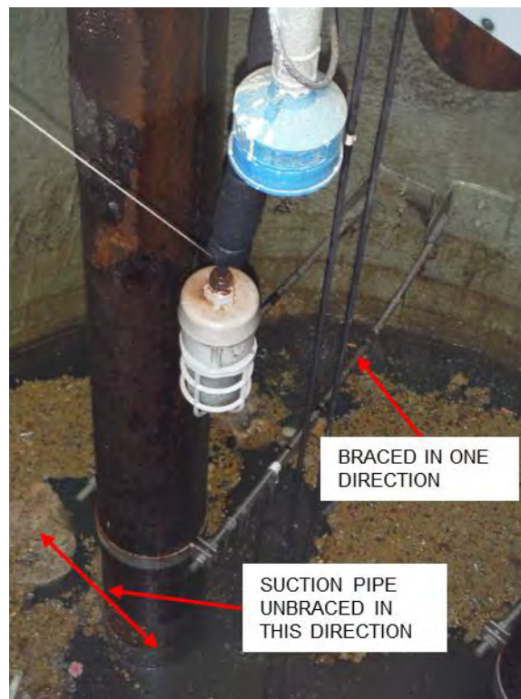
Figure 3.29 – Suction Pipes Only Seismically Braced in One Direction
