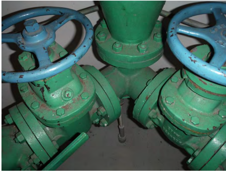
Figure 3.9 – Valves and Pipes not Seismically Braced
