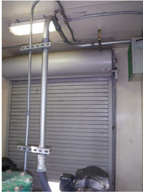
Figure 3.31 – Large Diameter Conduit does not Appear to be Adequately Braced
