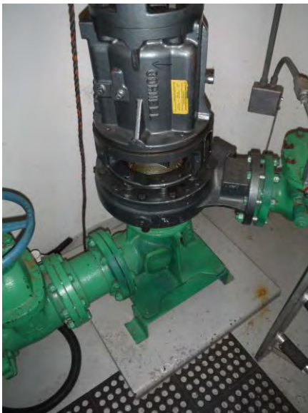
(a) East Pump Assembly
