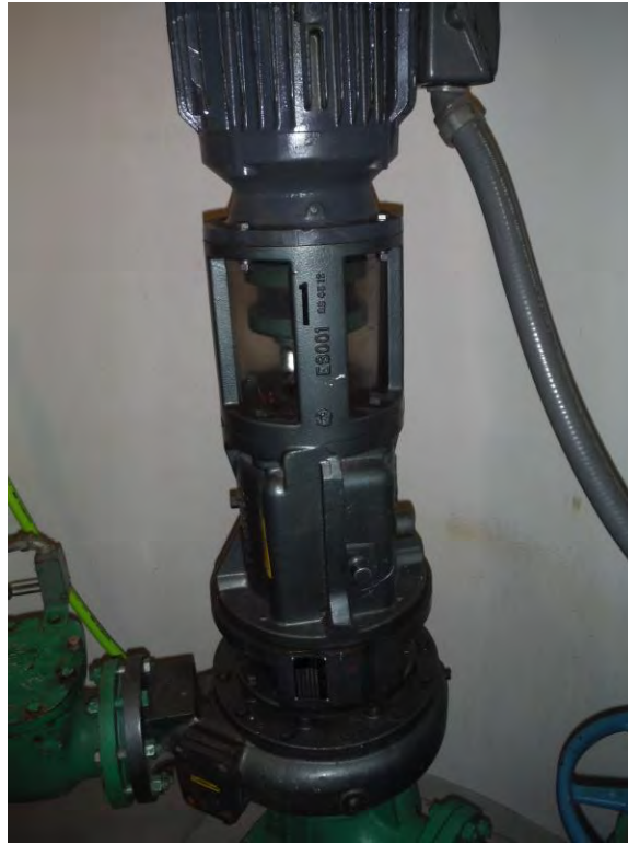
Figure 3.11 – Pump Assembly not Braced to Structure Above Center of Gravity
