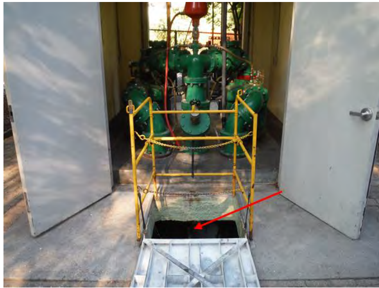
Figure 3.22 – Wet Well Access
