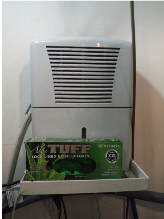
Figure 3.13 – Unrestrained Dehumidifier Unit
