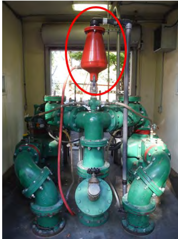
Figure 3.30 – Air Can does not Appear to be Adequately Seismically Braced
