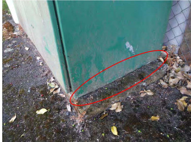
(b) No Anchors between Cabinet and Concrete Pad Visible from Exterior of Cabinet
