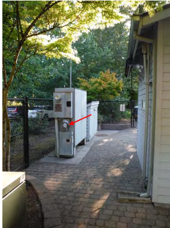
Figure 3.20 – Emergency Generator Hookup on Electrical Cabinet
