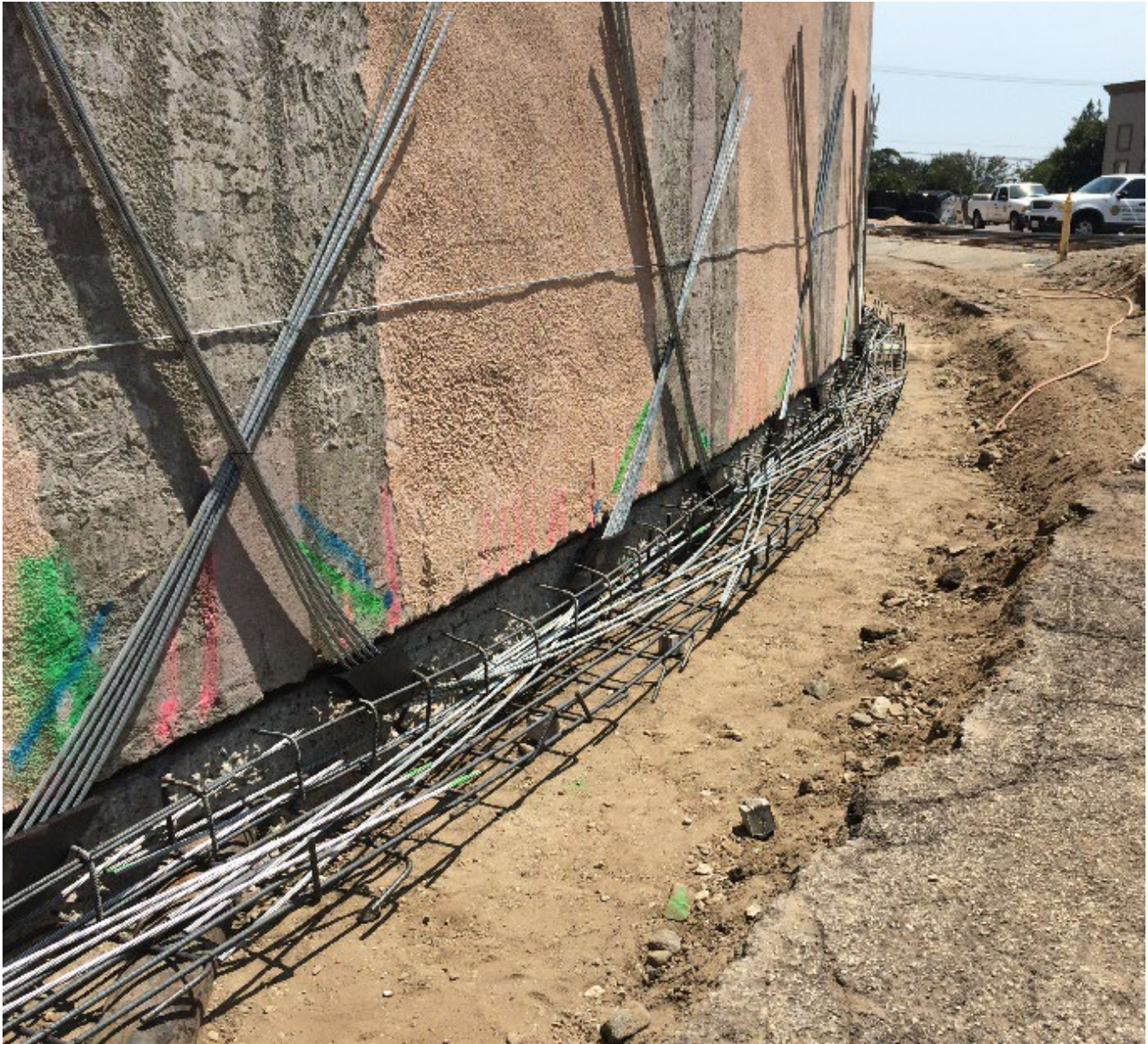
Figure 8-3. Seismic Cables Installed on an Existing Concrete Tank
