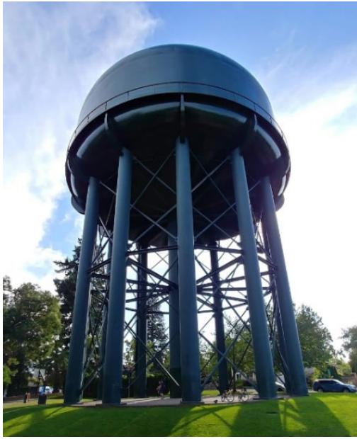
Figure 8-1. Elevated Water Tower
