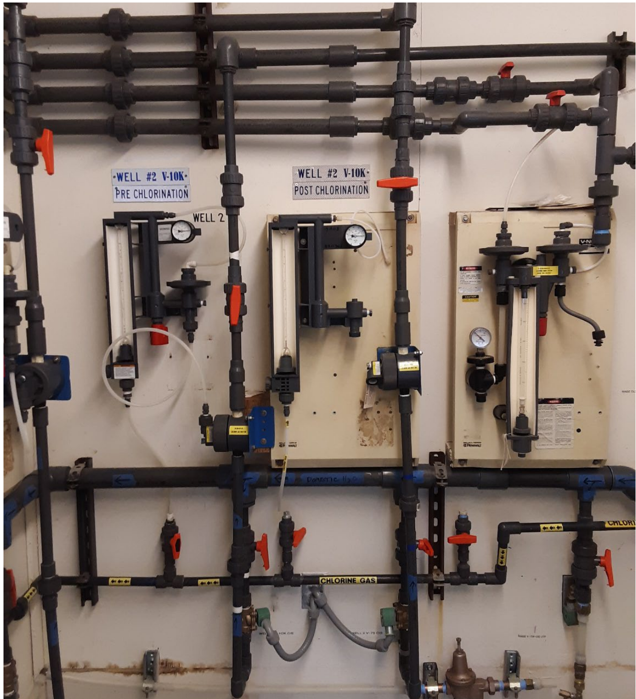
Figure 2-3. Chemical Feed Piping
