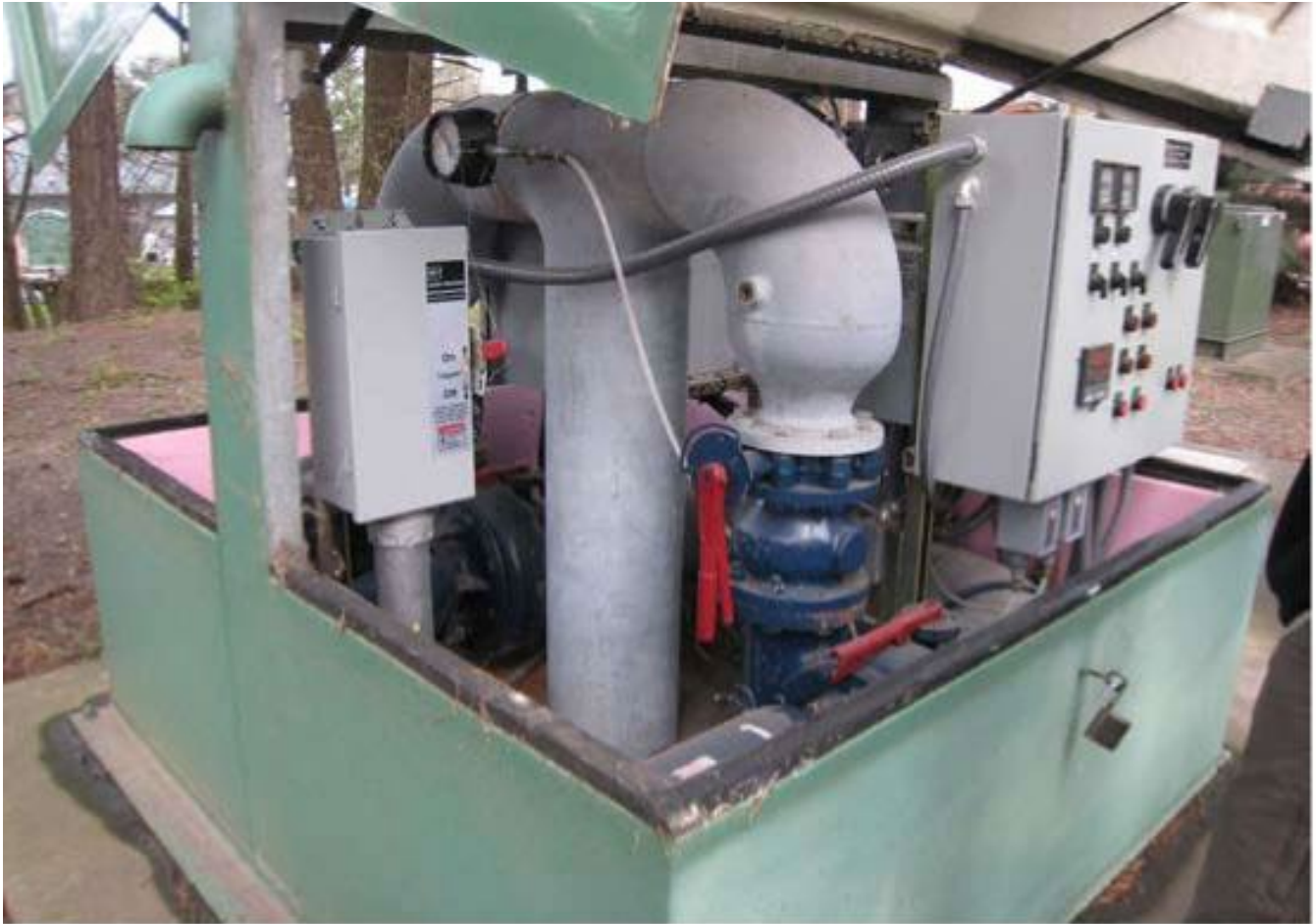
Figure 5-1. Clackamas River Water Intertie Pump Station
