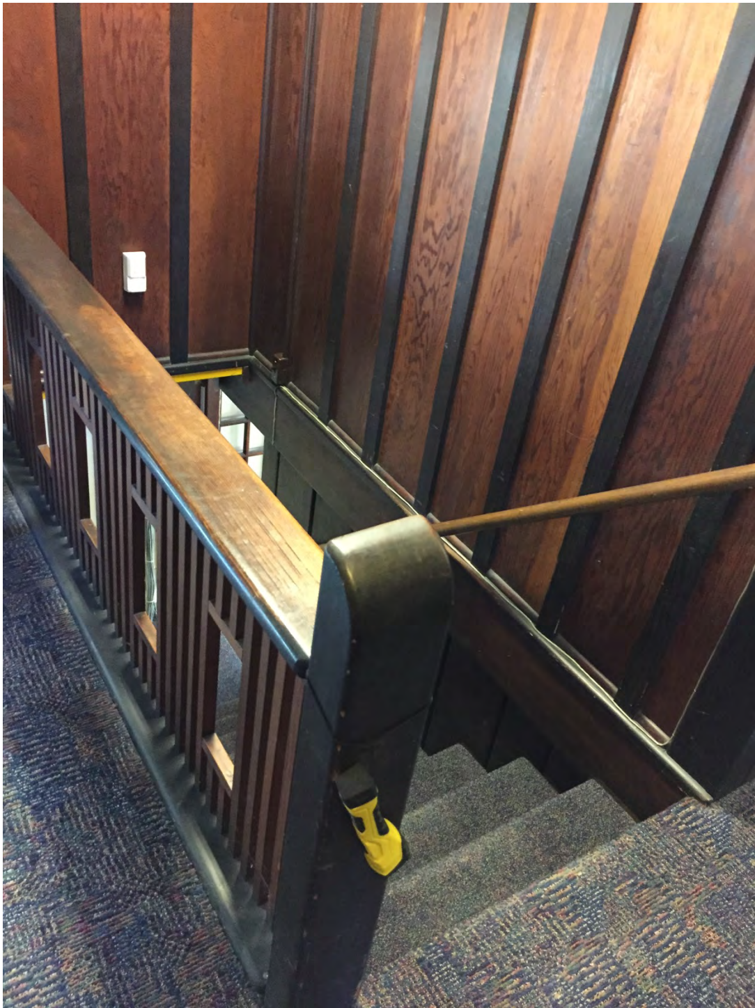
12. Interior view at upper level of c. 1906 structure, looking downstairs and southwest.
