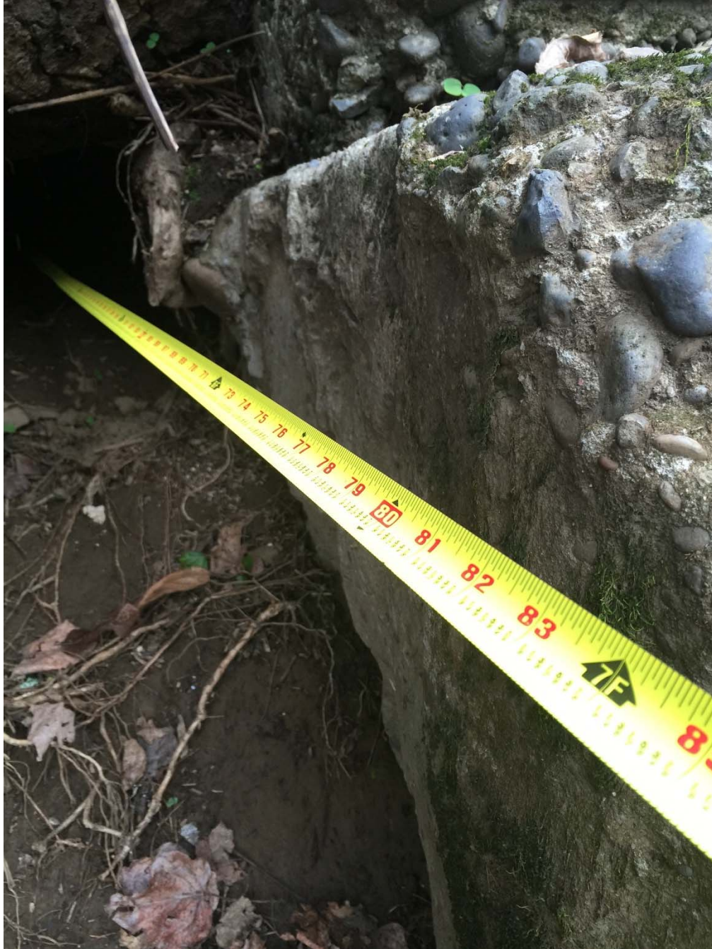
Possible Animal Hole – North Abutment West Corner Hole is 72 Inches Deep One of Two Holes
