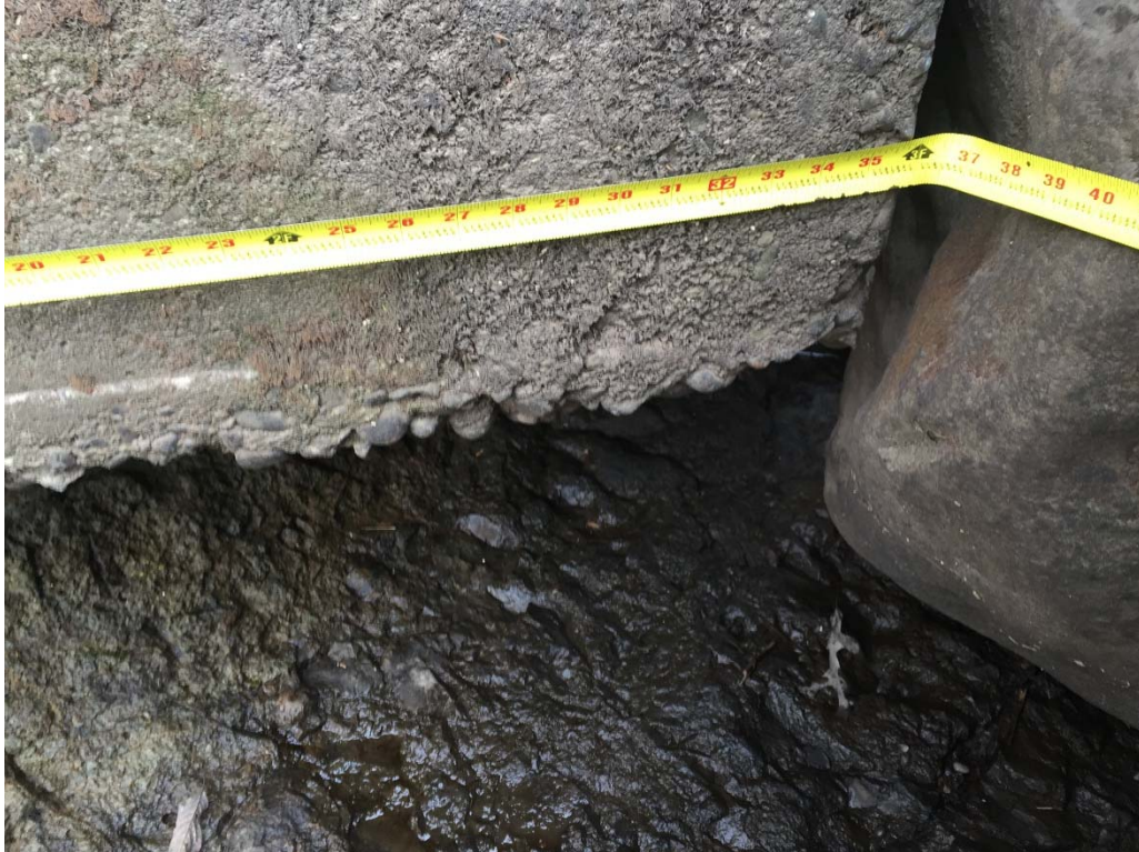
North Footing SW Corner (by boulder) – Scour Width
