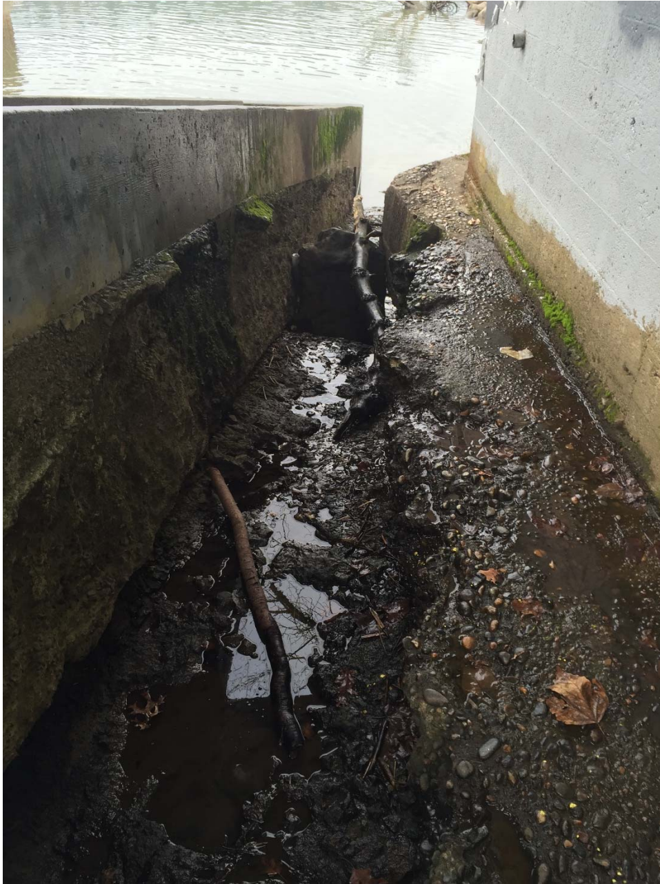
North Footing between Fish Ladder and Footing This area is 237 inches long
