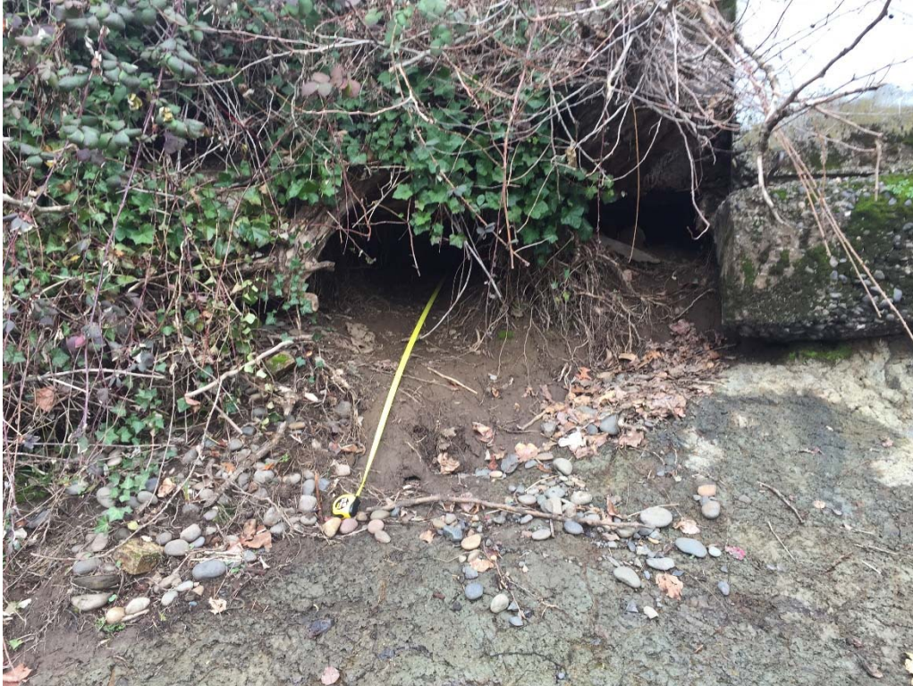
Animal Holes – North Abutment, West Side
