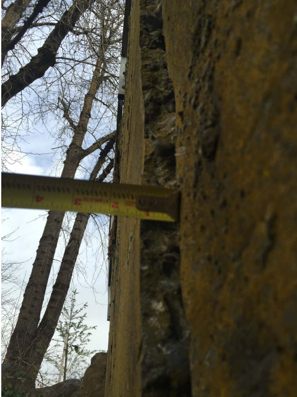
Wall Pushed Out (West) 1 to 1.5 inches
