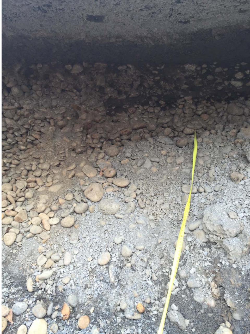
Looking at Undermining South Approach
