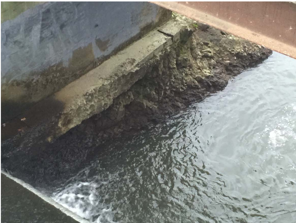
South Concrete Footing – Poured on Rock Undermined Maximum 8 inches (No Foundation Piles Visible)
