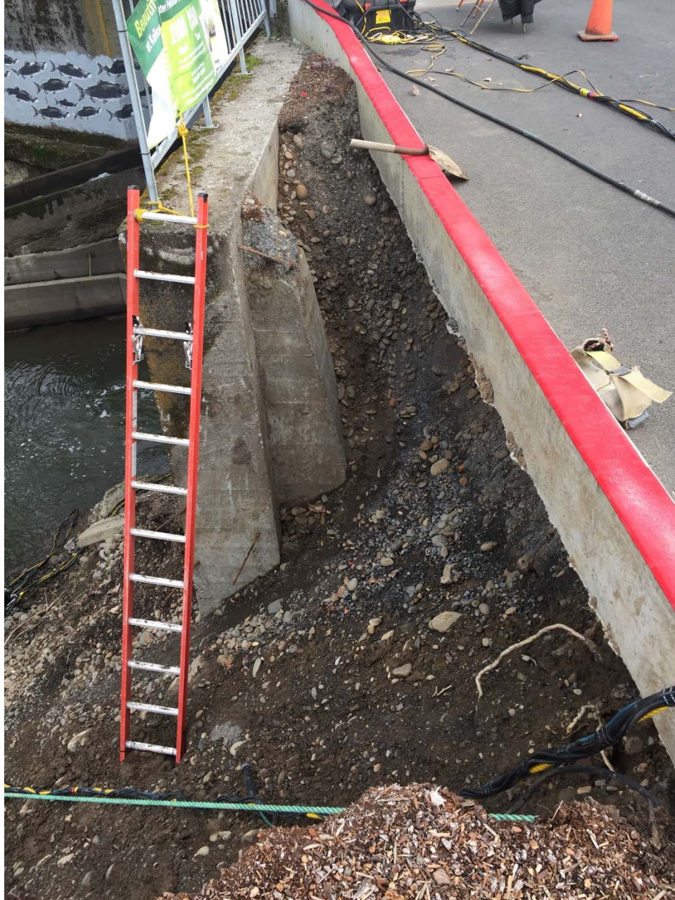
Undermining – South Abutment (Approach) West Wingwall in Foreground
