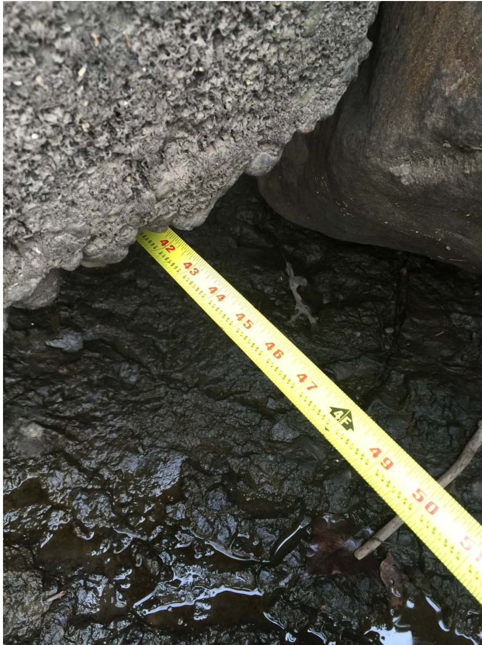
North Footing – SW Corner (by lodged boulder) Scour depth 42 inches x 36 inches wide
