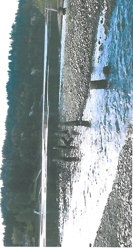
Photo 6. Pilings at the mouth of Johnson Creek (08/1673-1). The view is to the west.
