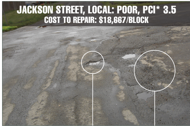
Poor drainage allows water to saturate base and sub-base.
