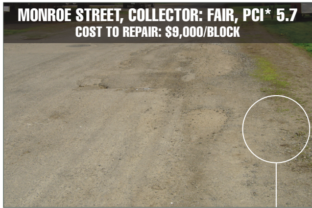
Poor shoulder drainage contributes to deterioration of aging asphalt. As asphalt is eroded, gravel is exposed and released.
