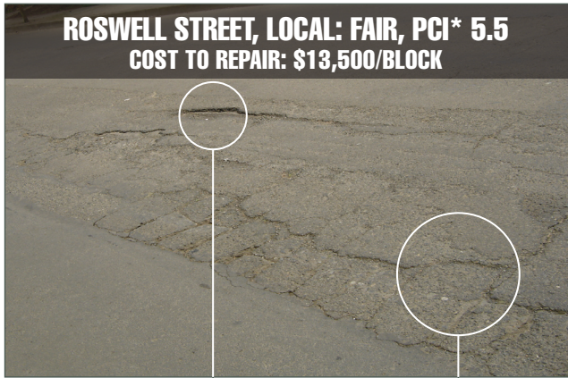
Water enters sub-base through cracks and, over time, the asphalt becomes brittle and breaks away.
