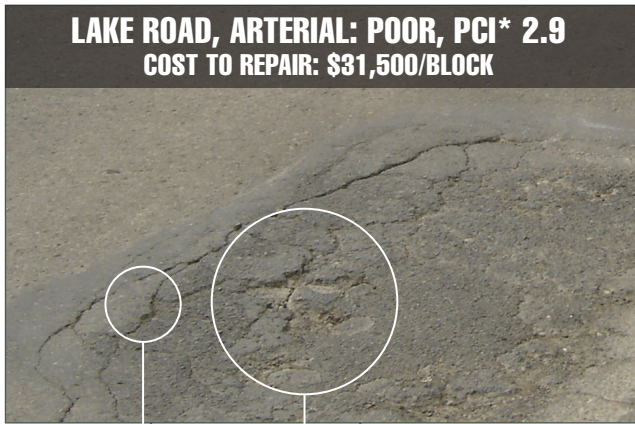
Cracks due to aging.
