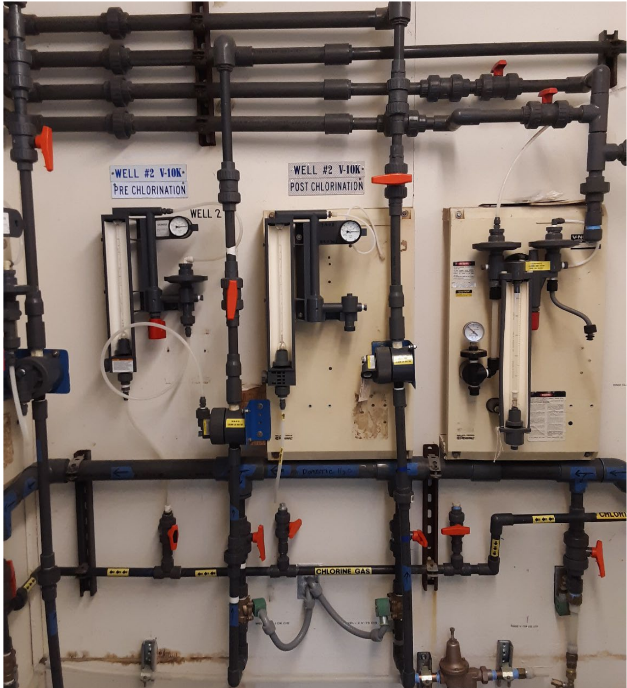
Figure 2-3. Chemical Feed Piping
