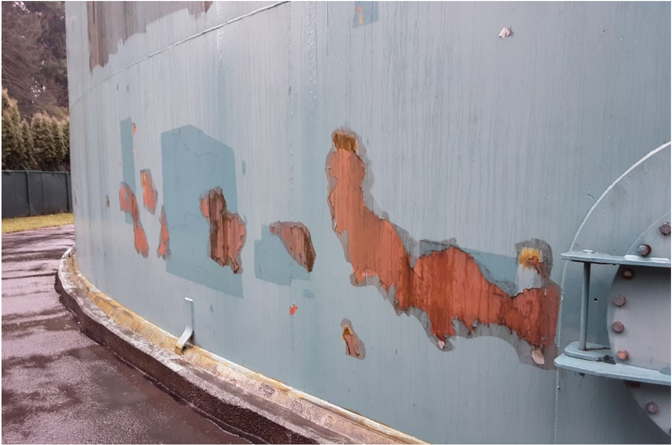
Figure 2-1. Stanley Reservoir Exterior Paint Condition
