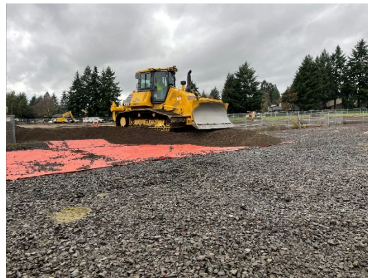
11/19/21 Parcel 2 entrance at West of Parcel 2, showing orange demarcation geotextile in proposed landscaping areas.
