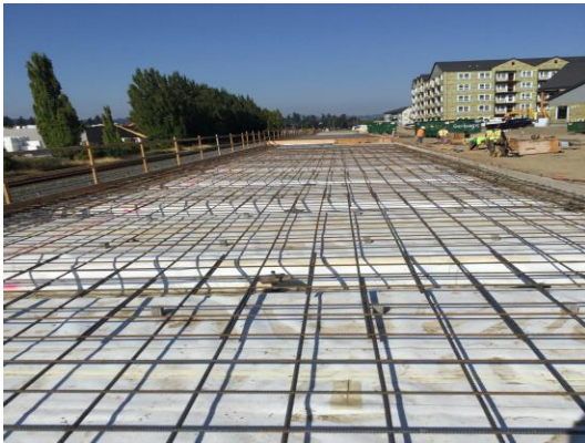
10/3/22 Parcel 2 Garage 2 rebar over vapor barrier prior to slab-on-grade pour, viewing northwest.
