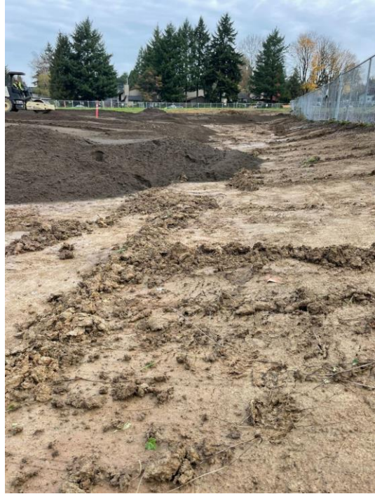
11/10/21 Parcel 1 fill nearing Parcel 2's fence, northward view from southern portion of Parcel 1. Cone in background marks sewer manhole.
