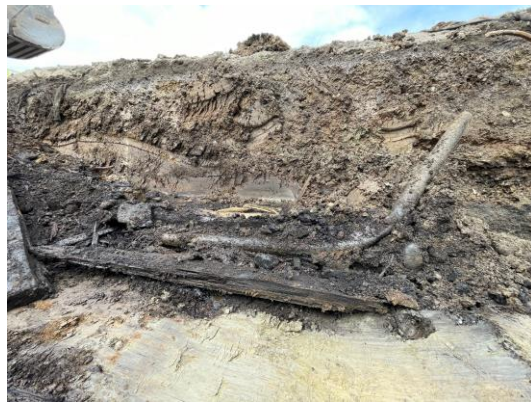
6/2/22 Historical piping and wood unearthed during excavation for Garage 2 retaining wall. Wood, piping, and stained soil were segregated out and separately stockpiled.
