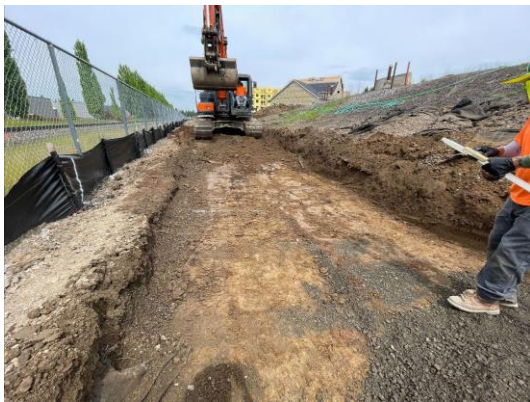
6/1/22 Garage 2 retaining wall foundation excavation (Parcel 2), looking west, along southern property line. Railroad to left.
