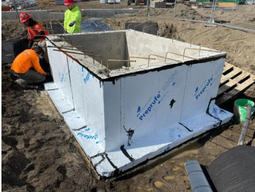
3/16/22 Post-applied PrePrufe 800PA vapor barrier installation on Clubhouse elevator pit stem walls by Sawtooth, with Bituthene Liquid Membrane.
