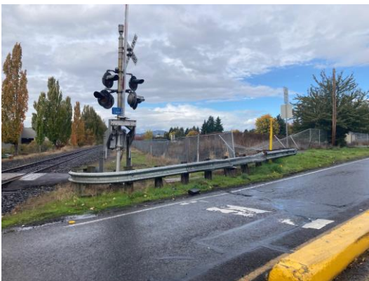
10/20/21 view of Parcel 2 from SE, showing a damaged area of southeastern perimeter fence, to be fixed on 10/25.
