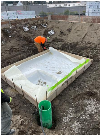
2/24/22 Parcel 2 Clubhouse elevator pit - PrePrufe 275 vapor barrier being placed over forms by certified installer Umqua.
