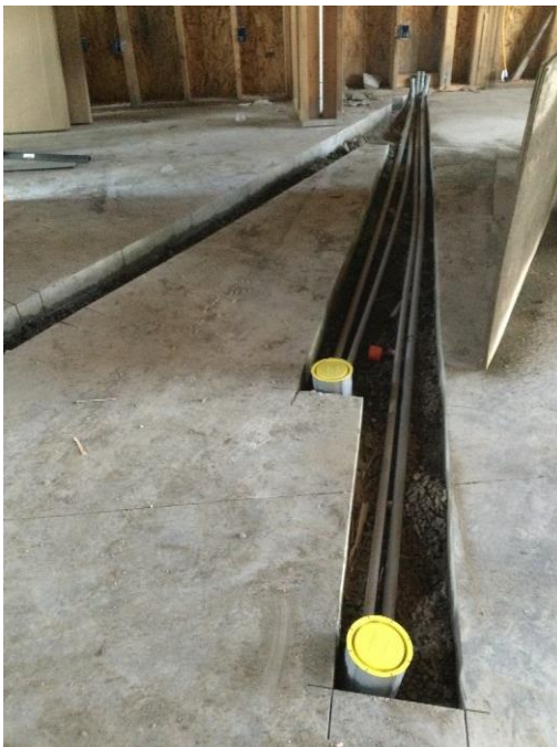
12/1/22 Parcel 2 Clubhouse slab and vapor barrier breach before repair.
