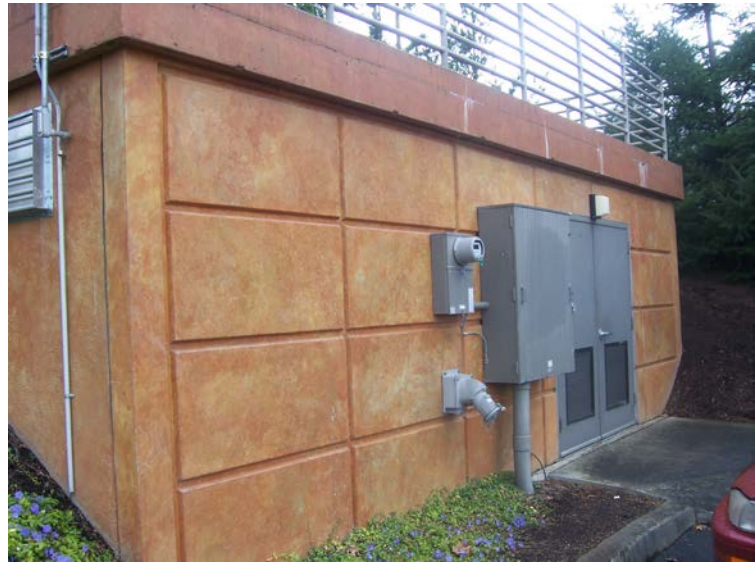
Figure 3-9. Lava Drive Pump Station
