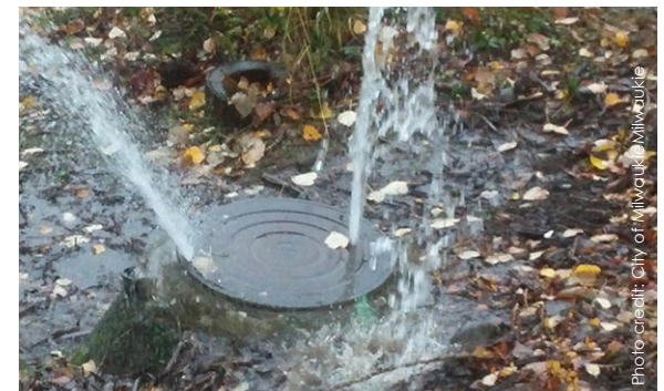
Storm drain surcharge in 2015
