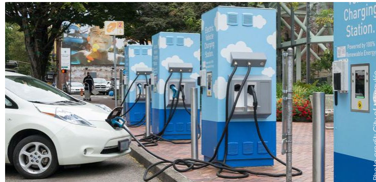
Electric vehicle charging station
