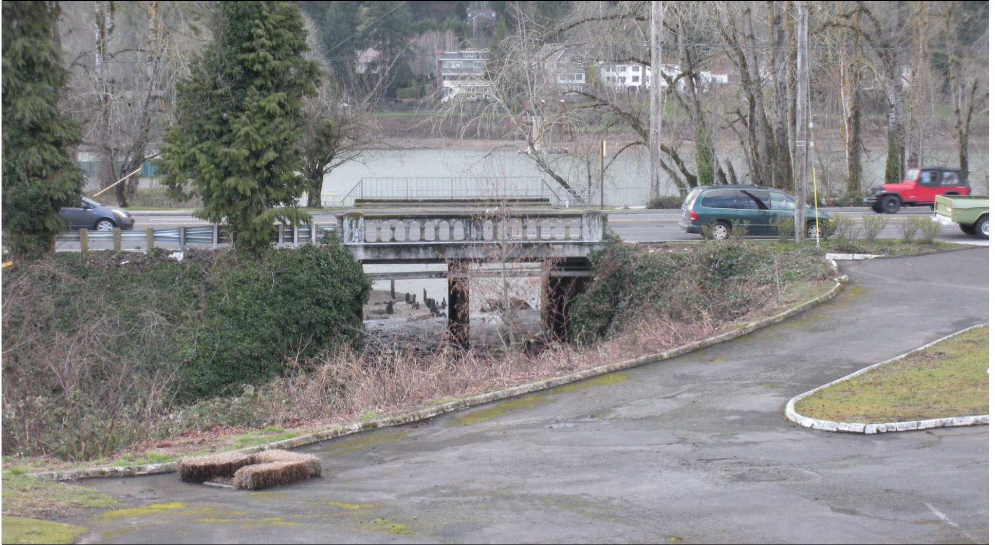
As you get closer, can see the Willamette both over and under the bridge – positive
