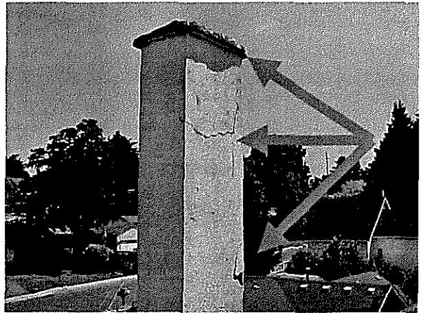
Cracked and chipped stucco on the fireplace chimney with deteriorated chimney cap.
