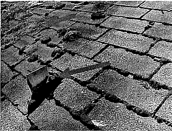
Poor roof shingle condition with moss build up and old hardware penetration through the shingles.
