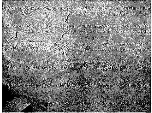
Basement interior wall skim coat deteriorated from moisture penetration.
