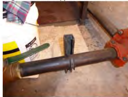
Fig. 4 – Pit oil line (lacks seismic overspeed valve)
