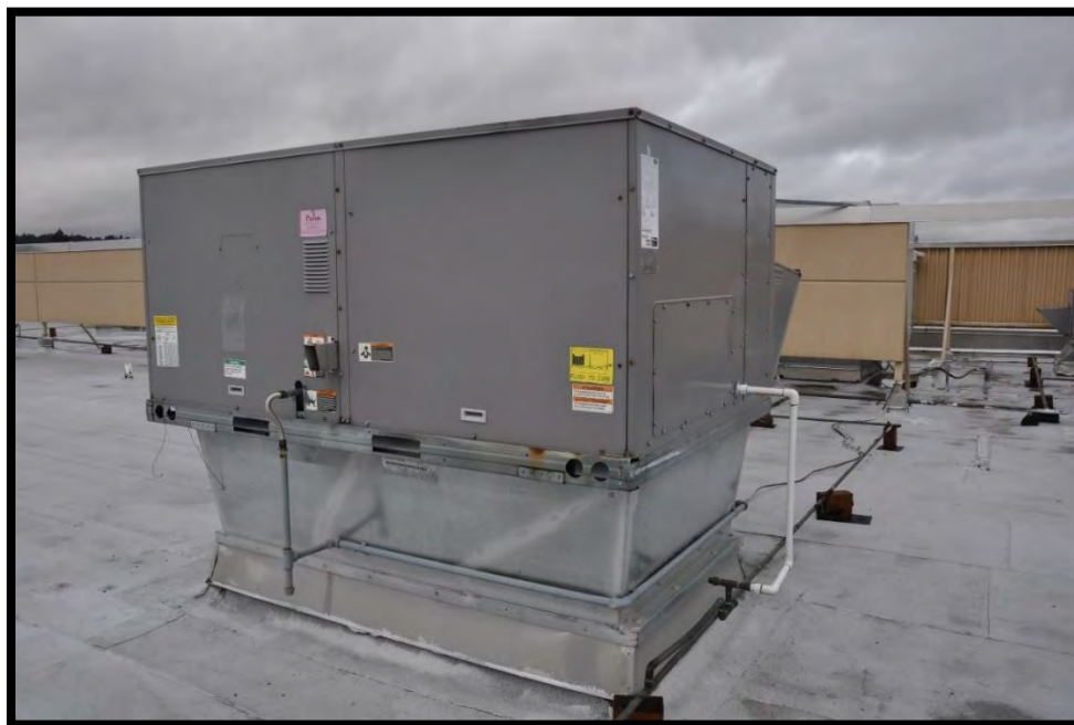
Figure 25: Example of Roof Top HVAC Equipment with Missing Anchorage to Curb
