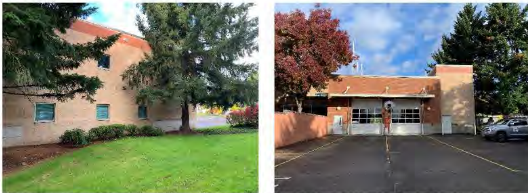
Photographs 1 and 2. East side (left) and south side (right) exterior of existing public safety building.
