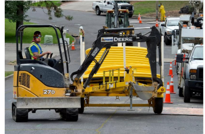
A new roll of natural gas line is driven into place for installation by WPI crews on Genesee Drive, Sept. 21, 2014, in Spokane. The Washington Building Code Council approved on Friday, April 22, 2022, significant restrictions on the use of natural gas in new commercial buildings. (DAN ROLLO/The Spokesman-Review)
