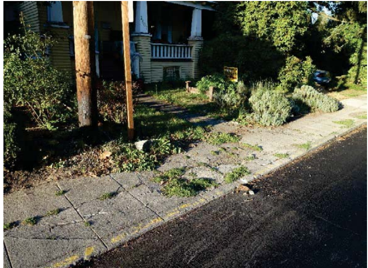
Example of deteriorating sidewalk condition on Monroe Street near 25th Avenue
