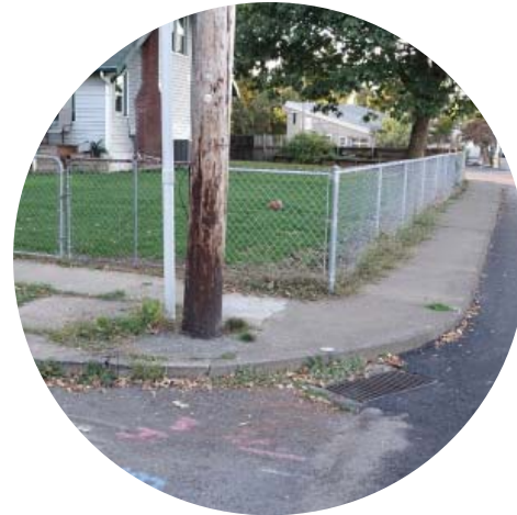
Intersections frequently lack curb ramps and other enhancements necessary for ADA compliance
