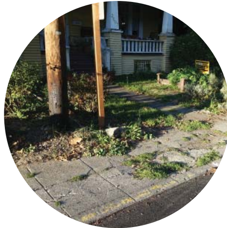
Sidewalks in this section are deteriorating in the vicinity of Spring Creek
